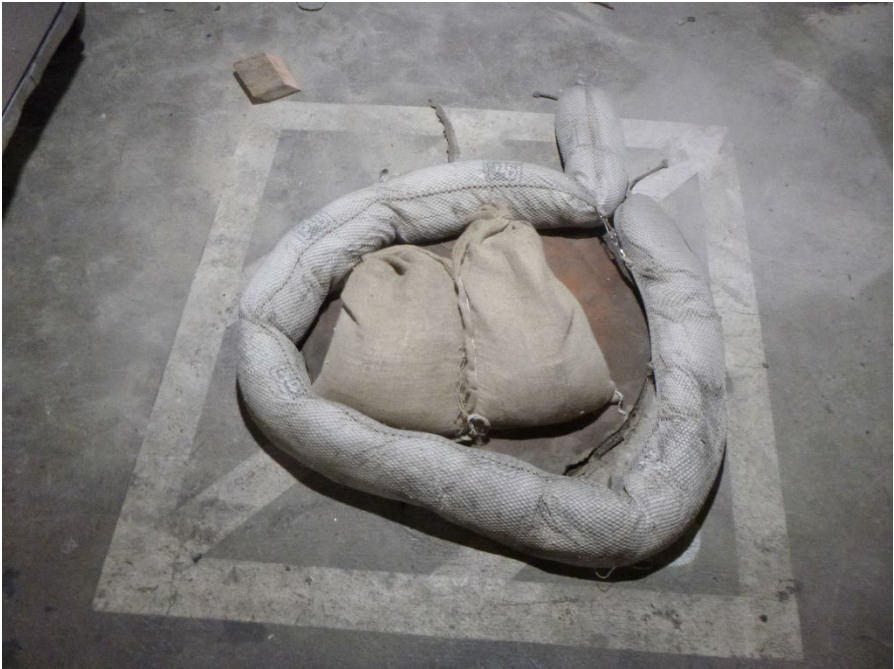
[P1040796.JPG] – RHMW03 Seal (Before Sampling) – 10/22/2024 – 0909
