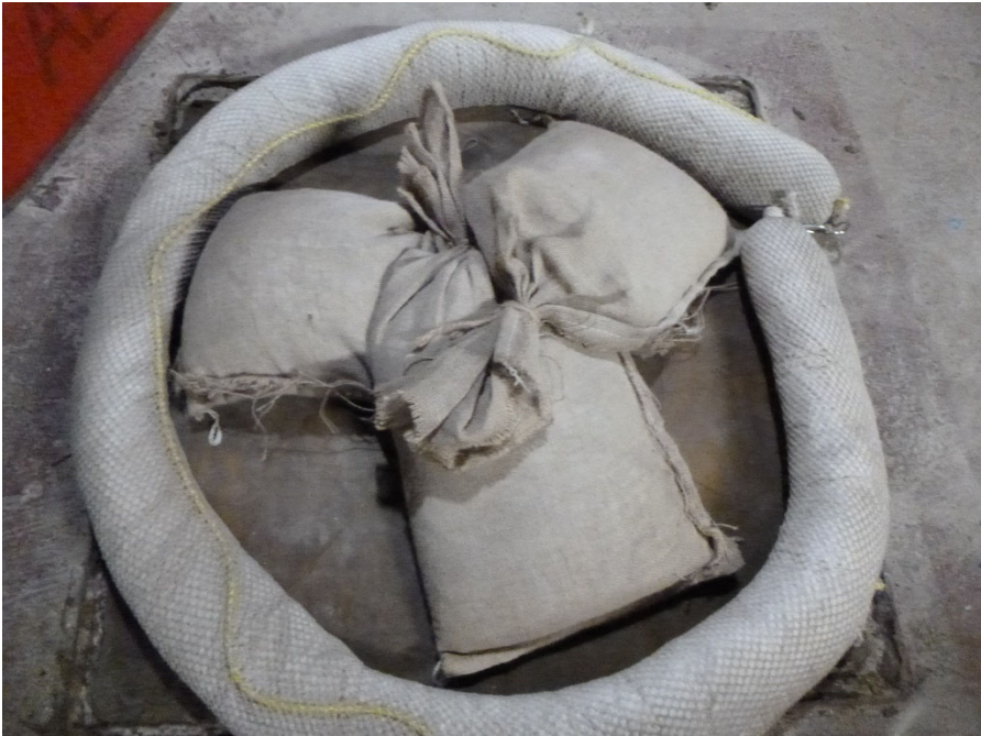
[P1040607.JPG] – RHMW05 Seal (Before Sampling) – 8/21/2024 – 1049
