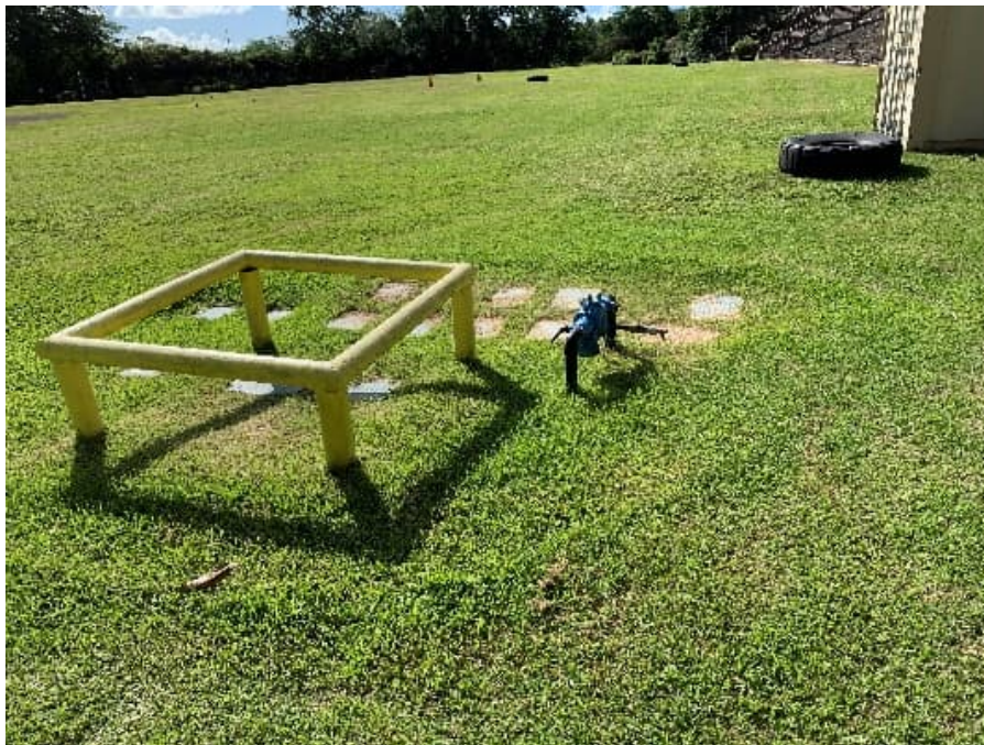
Photograph 47: Backflow Preventer and Valve Boxes
