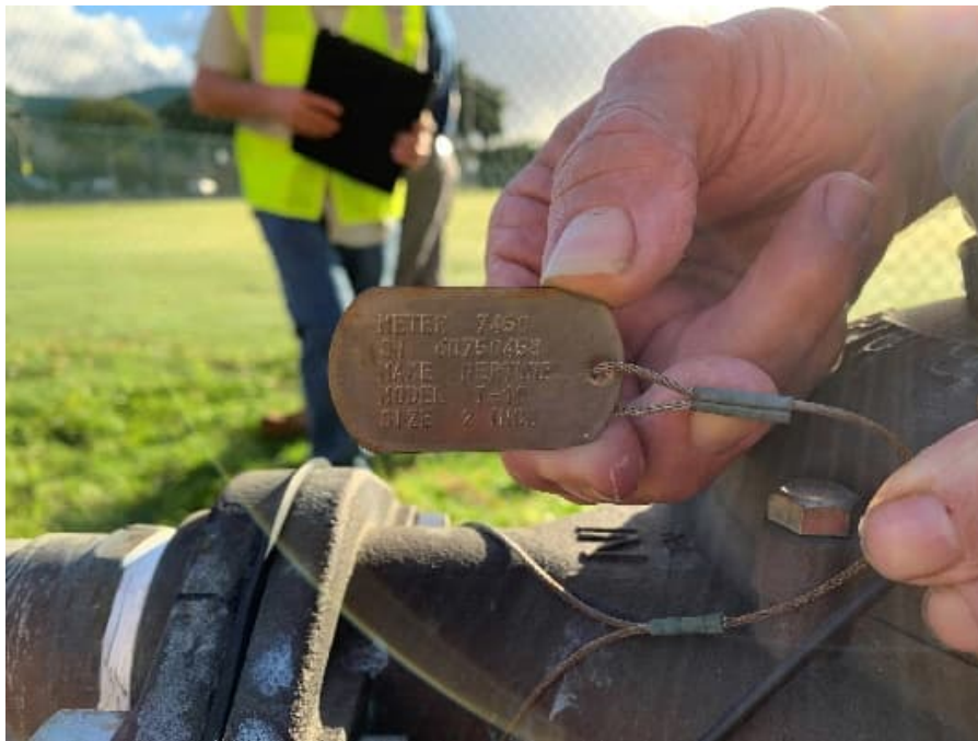
Photograph 8: Backflow Preventer ID Tag
