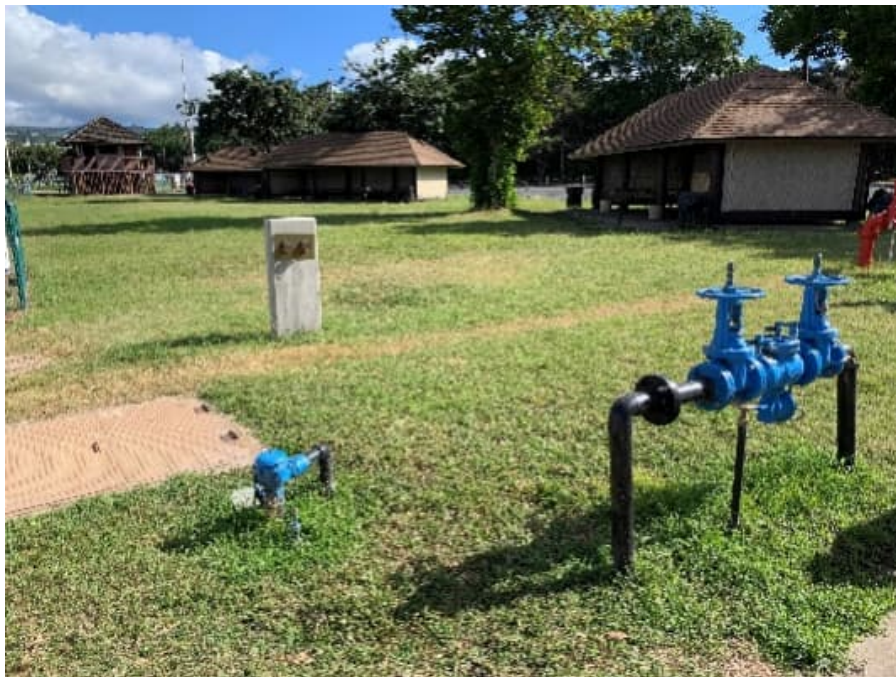
Photograph 58: Backflow Preventer near Cabanas and Restaurant 604
