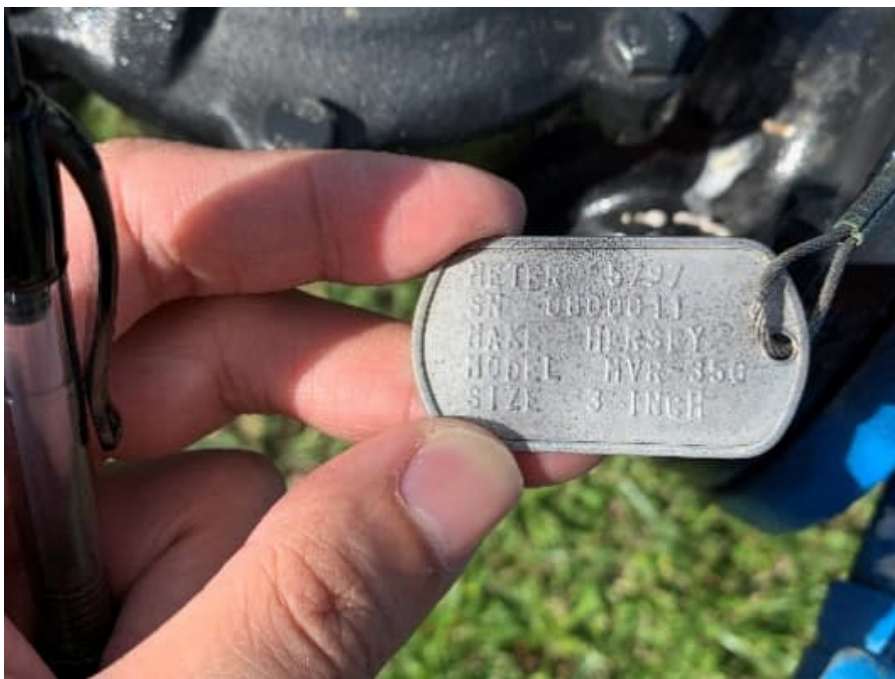
Photograph 64: Equipment ID Tags
