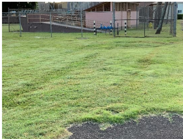
Photograph 2: Location of Backflow Preventer
