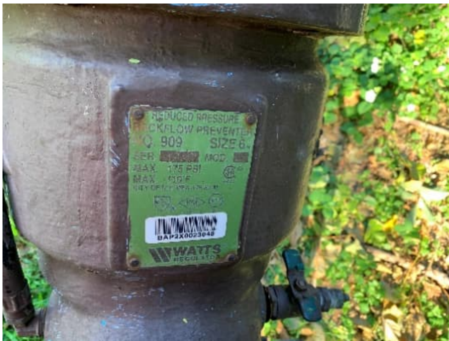
Photograph 21: Backflow Preventer ID Tag
