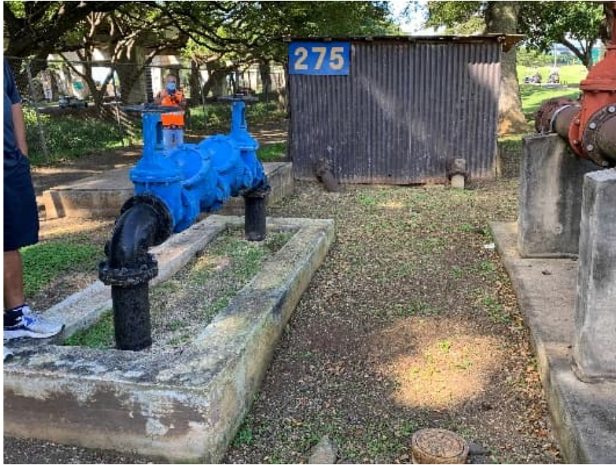
Photograph 76: Inactive Backflow Preventer
