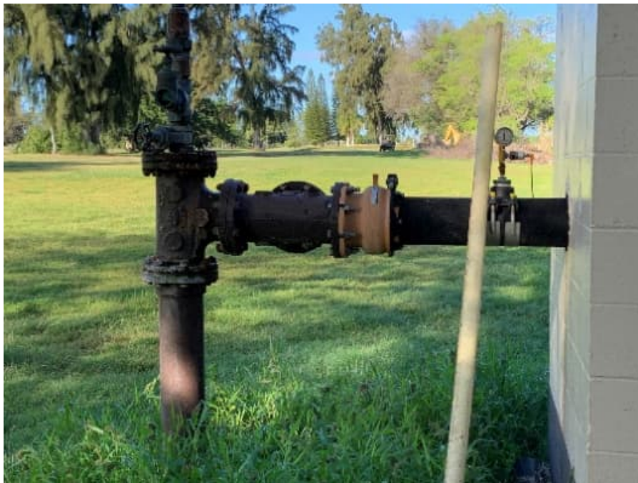
Photograph 23: Piping Exiting Building 3574
