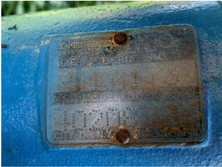
Photograph 11: Backflow Preventer ID Tag
