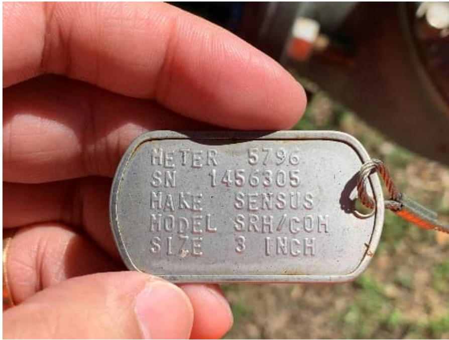
Photograph 75: Equipment ID Tag, Backflow Preventer across from the A-Frame
