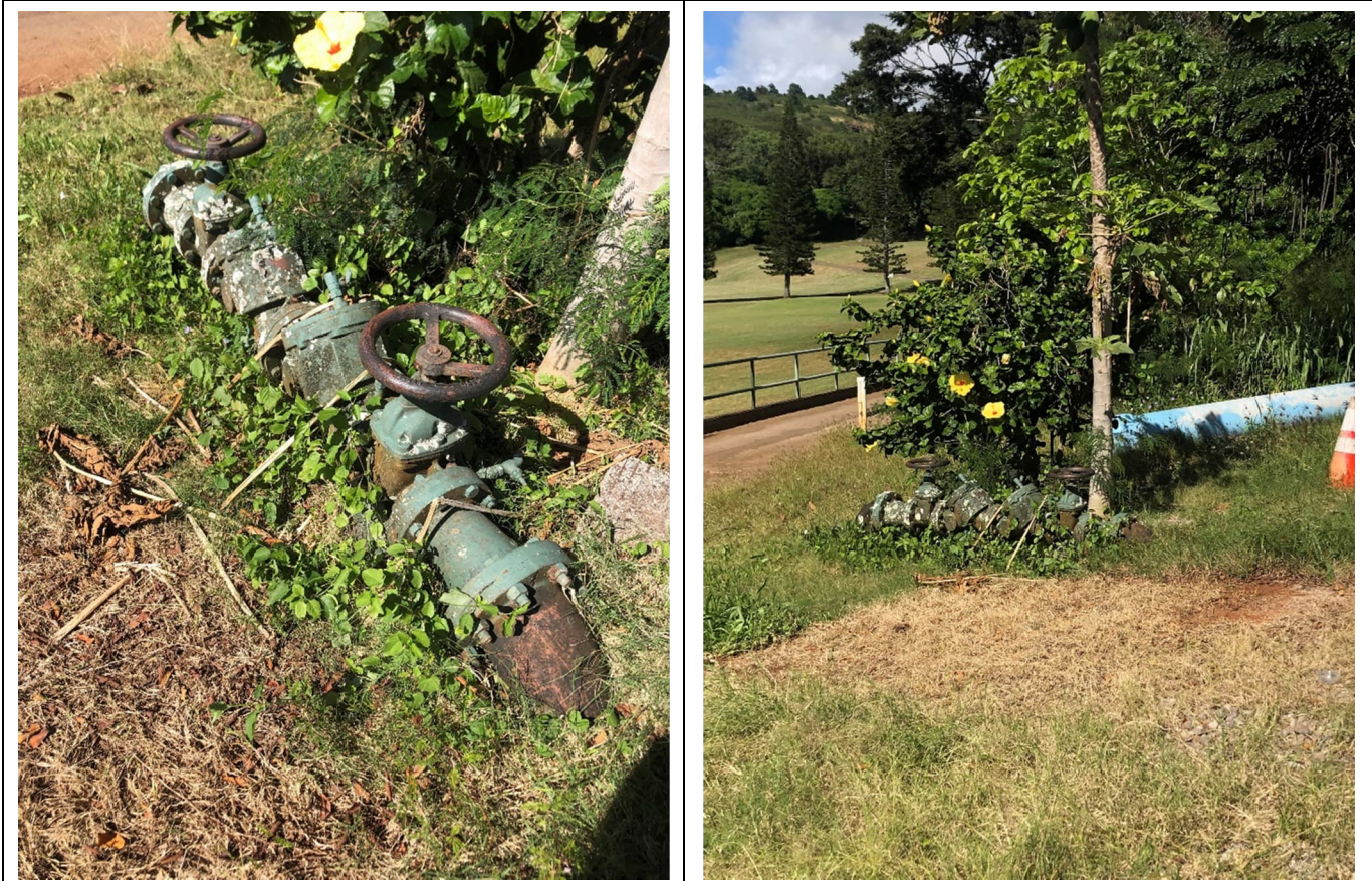
Photograph 1: Active Backflow Preventer, close up
