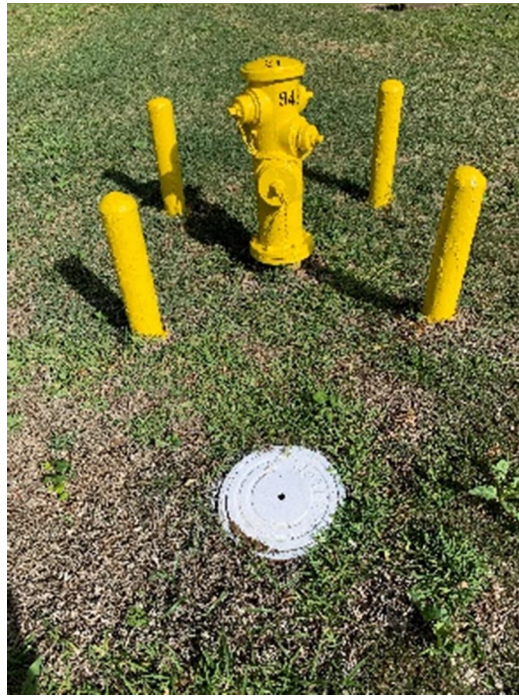
Photograph 46: Fire Hydrant and Valve Box
