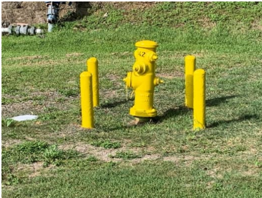
Photograph 41: Fire Hydrant near Connection
