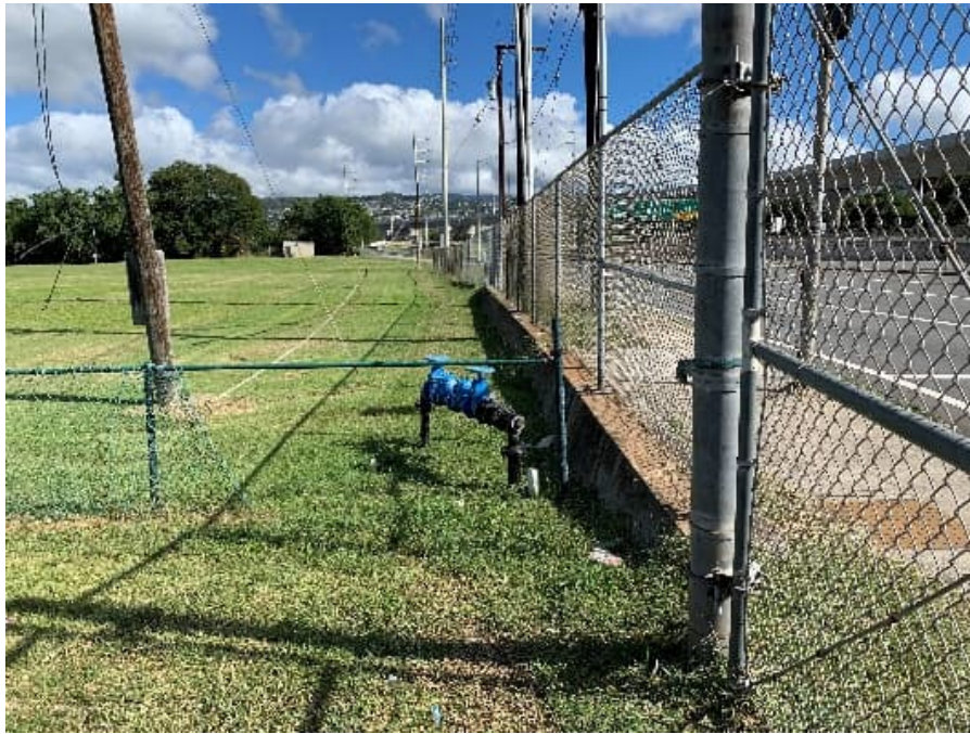
Photograph 67: Backflow Preventer location in relation to Highway
