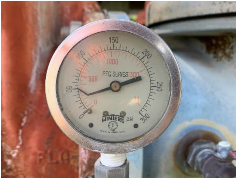
Photograph 78: Pressure Gauge on Active System
