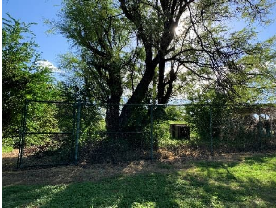
Photograph 26: Area Near Pumps and Transformers
