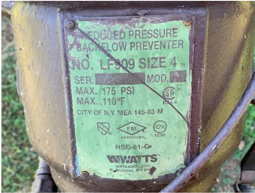
Photograph 32: Backflow Preventer ID Tag
