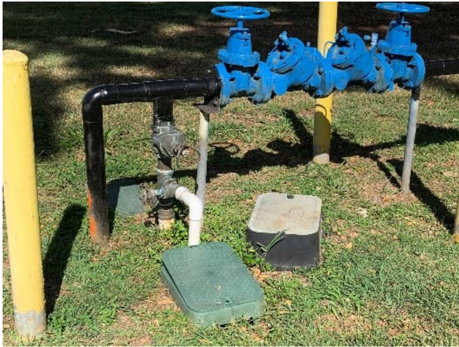
Photograph 73: Backflow Preventer across from the A-Frame
