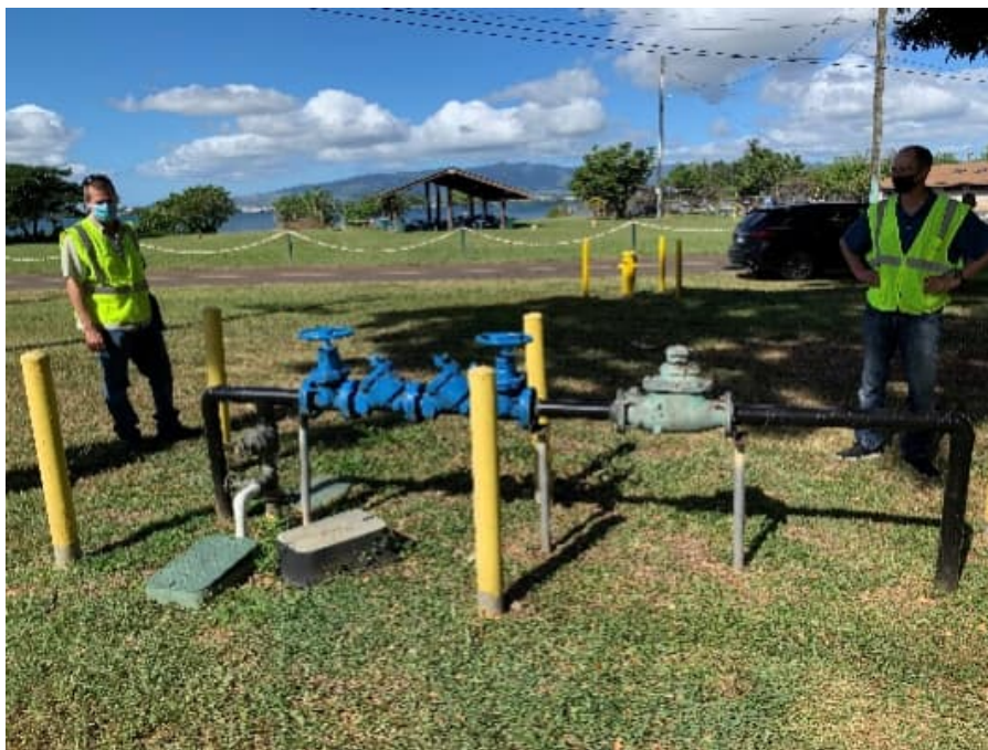
Photograph 72: Backflow Preventer across from the A-Frame
