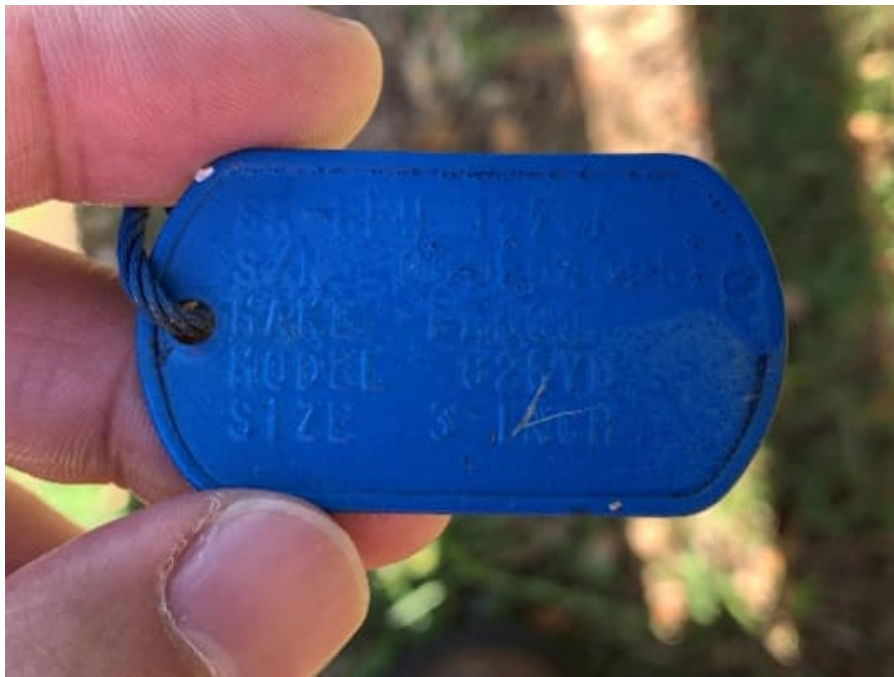
Photograph 74: Equipment ID Tag, Backflow Preventer across from the A-Frame
