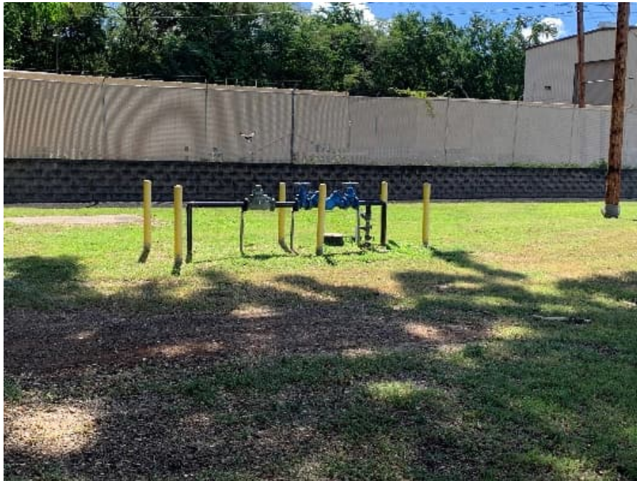
Photograph 71: Backflow Preventer across from the A-Frame
