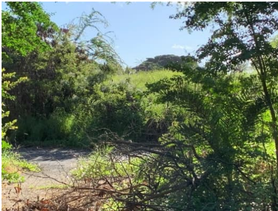
Photograph 27: Overgrown Holding Pond
