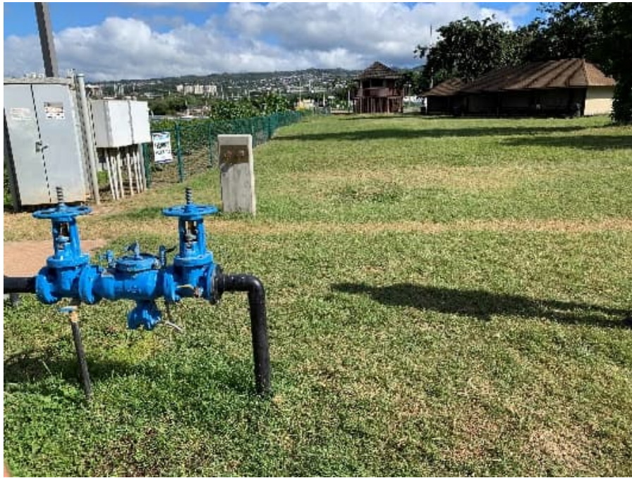
Photograph 57: Backflow Preventer near Cabanas and Restaurant 604
