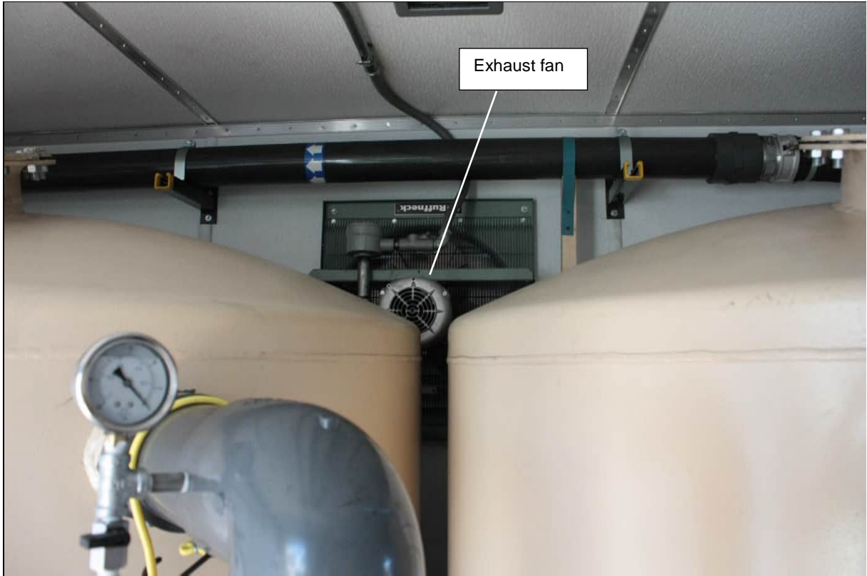
Photo 9. Location of exhaust fan in treatment room
