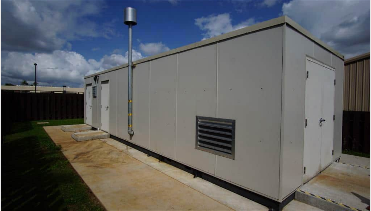
Photo 1. SVE system building
