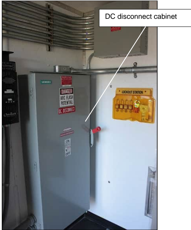
Photo 7. DC disconnect cabinet inside electrical room
