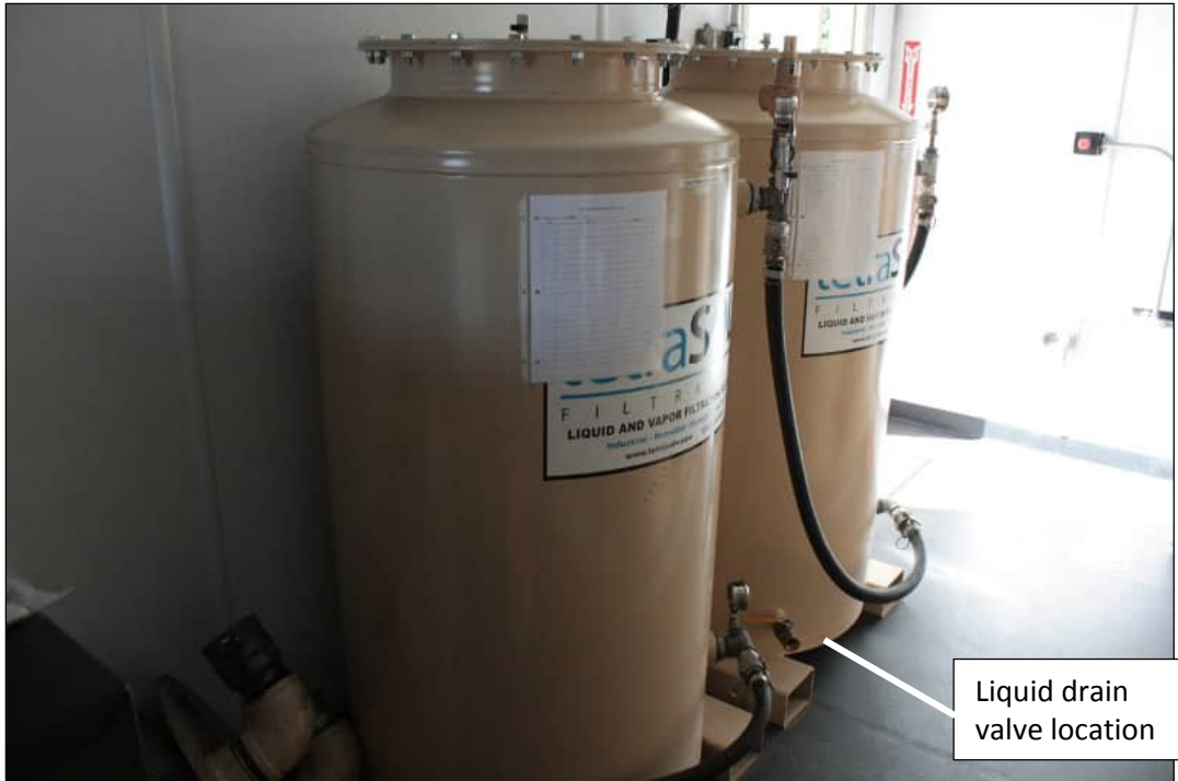
Photo 6. Valve location on an LGAC train vessel used to drain liquid before LGAC changeout.
