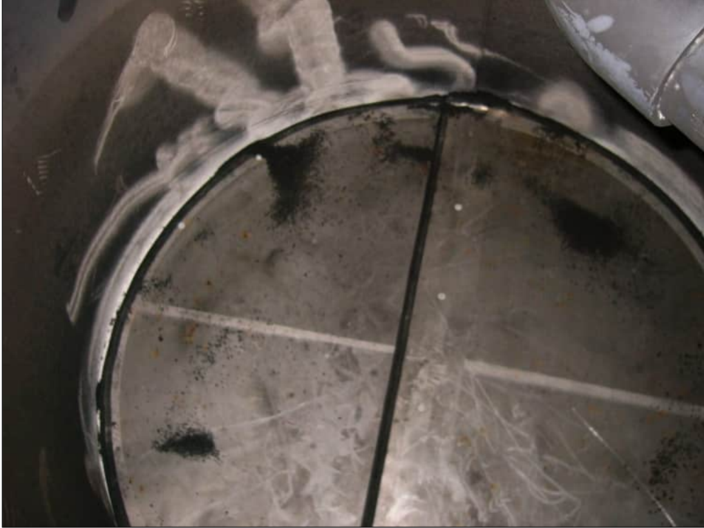
Photo 2. View inside a GAC vessel after all extractable spent carbon has been removed.
