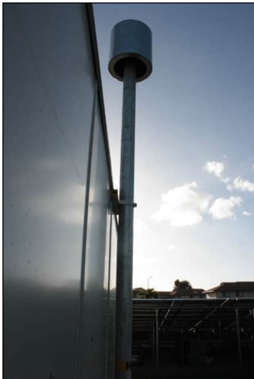
Photo 17. Exhaust stack on exterior of SVE system building with silencer
