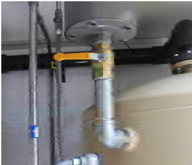
Vacuum Bleed Valve
