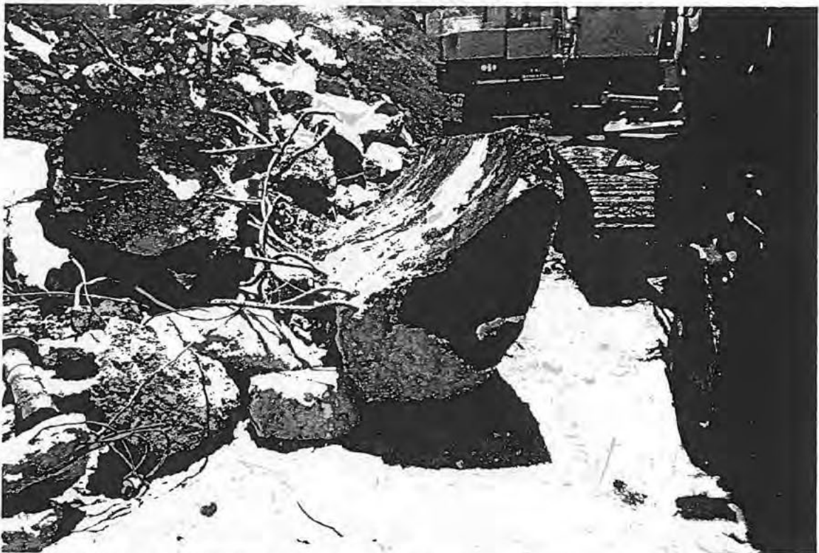
7 CUBIC YARDS CONCRETE BALLAST BLOCK ATTACHED TO VAULT AND ON TOP OF EACH TANK
