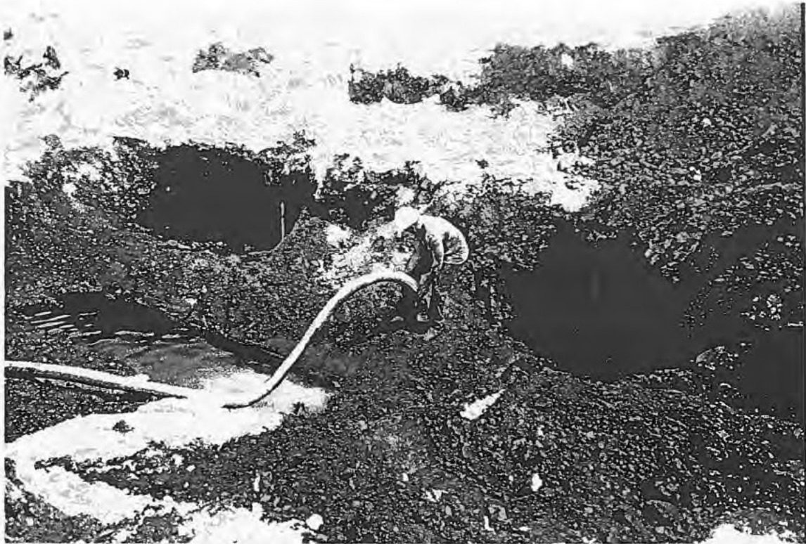
TANK EXPOSED AND CONTENTS BEING DRAINED. NOTE EXTENSIVE PULVERIZED COAL USED AS TANK AND PIPE BEDDING MATERIAL. FREE LIQUID IS TIDAL WATER TABLE
