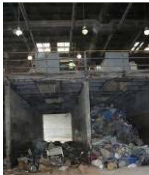
Photo 1-7. Elevated picking stations with bays underneath for separated material
