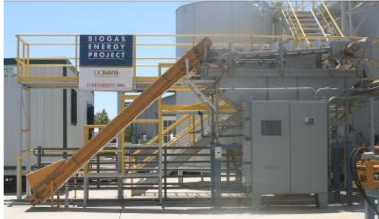
Photo 1-10. UC Davis Biogas Energy Project
