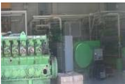
Photo 1-12. Engine generators using methane gas to produce electricity
