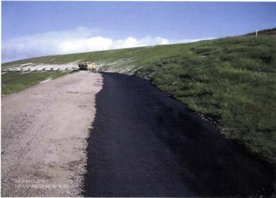
Photo 23 Installation of asphalt paved V-ditch along aggregate base surfaced landfill road. Note substantial vegetative establishment on the landfill cover.
