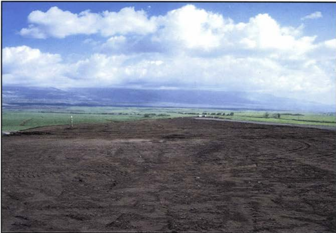
Photo 16 Completed MFC on top deck of landfill awaiting placement of soil-compost layer.
