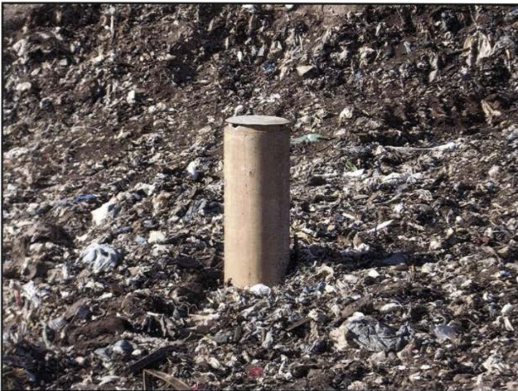
Photo 6 Excavation around newly installed 24-inch diameter concrete manhole riser pipe and foundation backfilled with compacted refuse.
