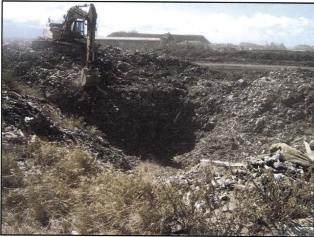
Photo 1 Excavation of leachate collection/drainage pipe to permit installation of new leachate collection and removal manhole riser.
