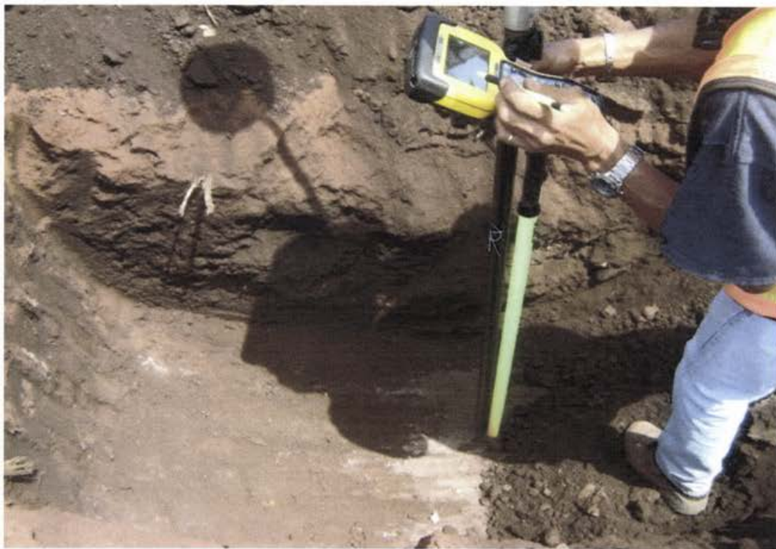
Photo 20 Surveying location of completed test pit for verification of Monolithic Final Cover (MFC).
