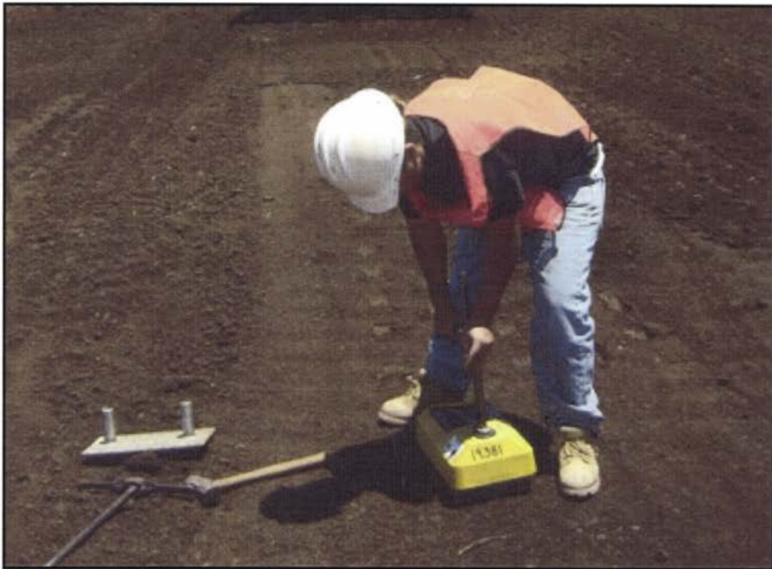
Photo 15 CQA monitor conducting field density and moisture content measurement on the compacted MFC soil using the Nuclear Gauge method (ASTM D2922).
