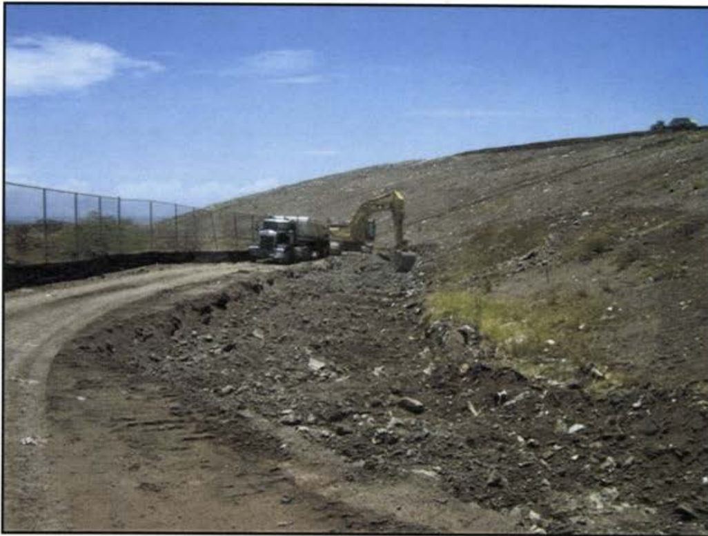
Photo 8 Excavating waste and interim cover soils to accommodate MCF soils and concrete trapezoidal drainage channel along perimeter road.
