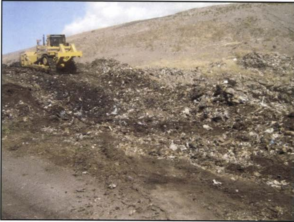
Photo 7 Relocating and regarding waste and interim cover soils to create drainage bench/road prior to placement of MFC soils.
