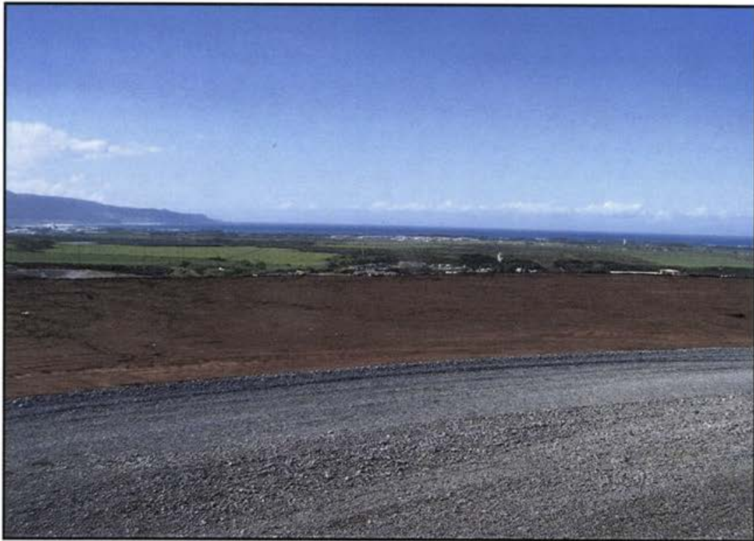
Photo 17 Completed MFC on top deck of landfill awaiting placement of soil-compost layer. Note aggregate base placed and compacted in preparation for asphalt concrete pavement.
