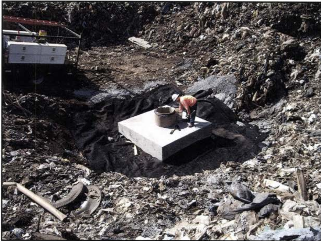
Photo 5 Foundation slab with forms removed. Worker preparing concrete manhole riser pipe for receipt of next segment of pipe.
