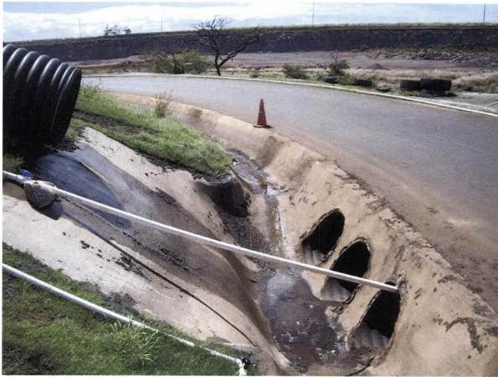
Photo 28 Collection point for perimeter channels and top deck drainage
