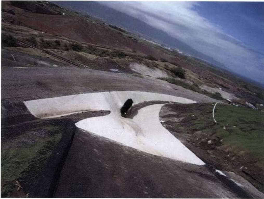
Photo 27 Collection point mid-slope bench and top deck drainage
