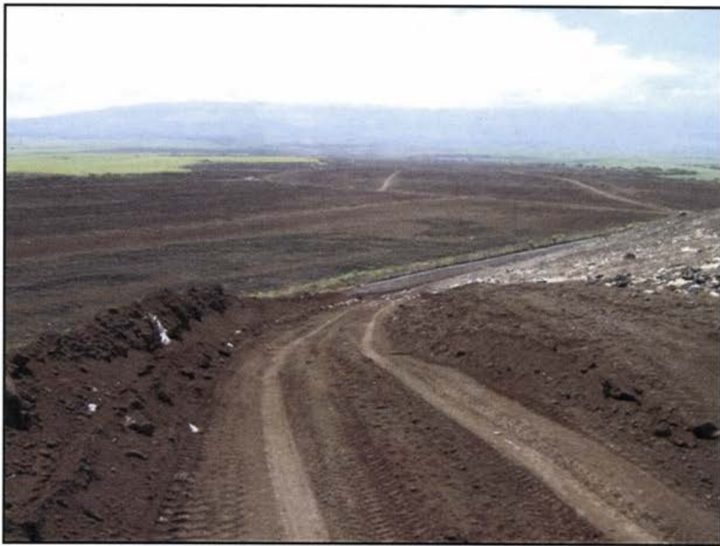
Photo 12 MFC soils placed, compacted, and rough graded on road from top of landfill to east side perimeter road
