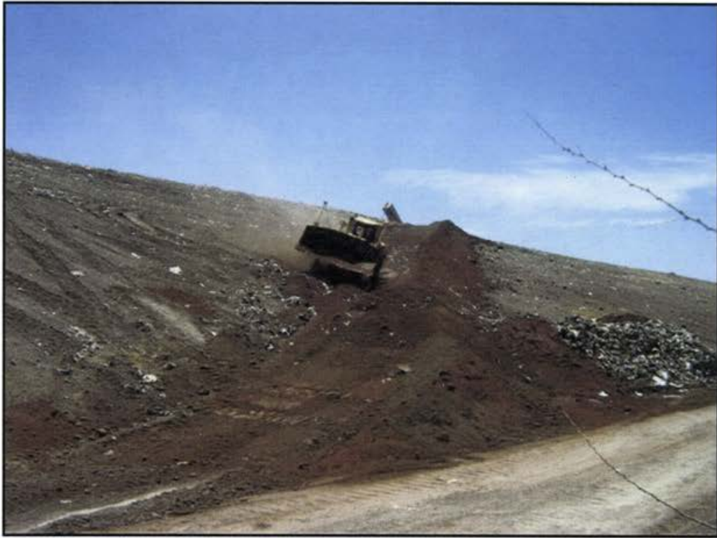
Photo 9 Relocating and regrading waste and interim cover soils to create drainage bench/road prior to placement of imported MFC soils.
