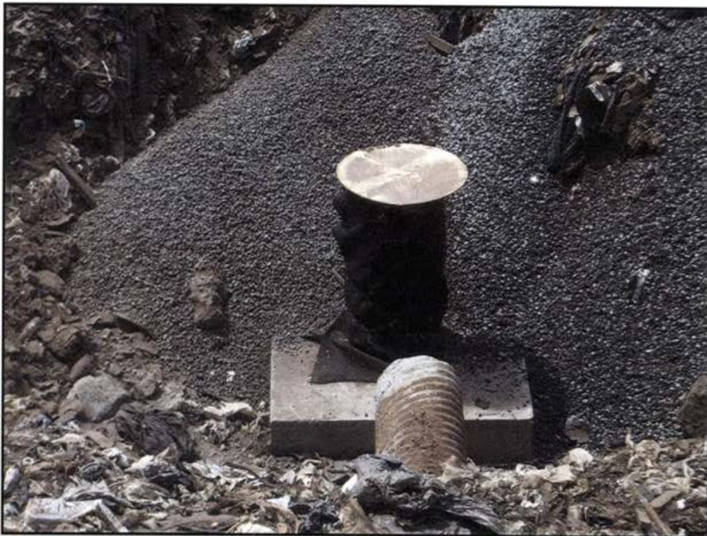
Photo 2 Steel-reinforced concrete foundation slab and 18-inch diameter perforated HDPE vertical inlet pipe with geotextile filter fabric wrapping. Note existing leachate drain pipe in foreground.
