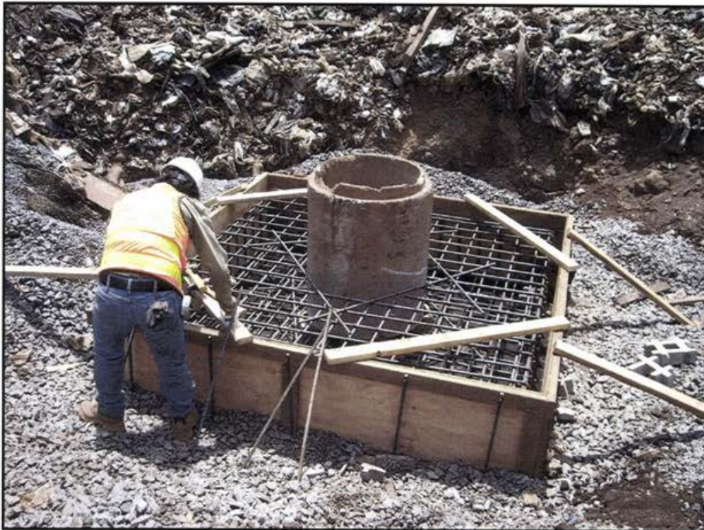
Photo 4 Installation of reinforcement steel and construction of concrete form in preparation to pour concrete foundation slab for the 24-inch diameter concrete manhole riser.
