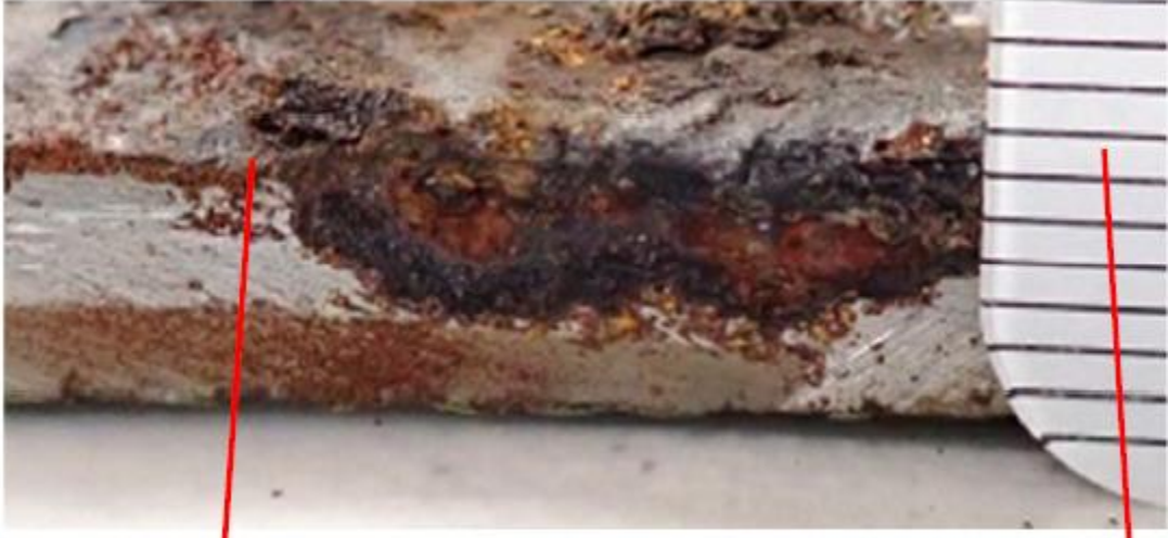
Figure 2: Image taken after coupon removal, prior to receipt by lab. What appears to be a deep corrosion pit was actually rust-covered staining of the edge surface.
