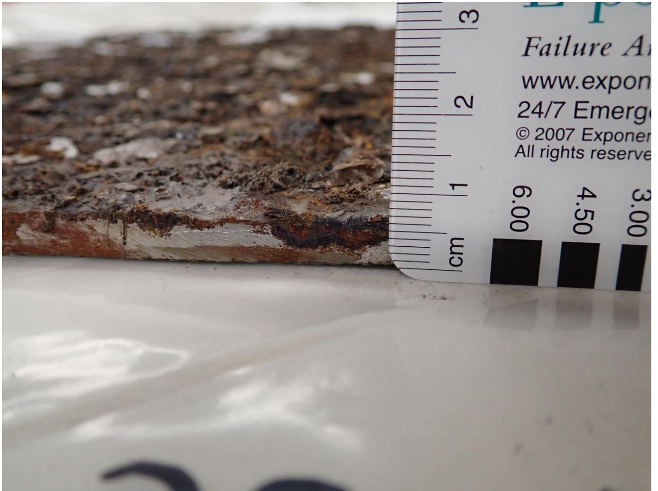
Figure 1: Edge of Coupon #7. Image from non-Navy source alleging the thickness of the remaining steel at the location shown alleging thickness less than the Navy's predictions.
