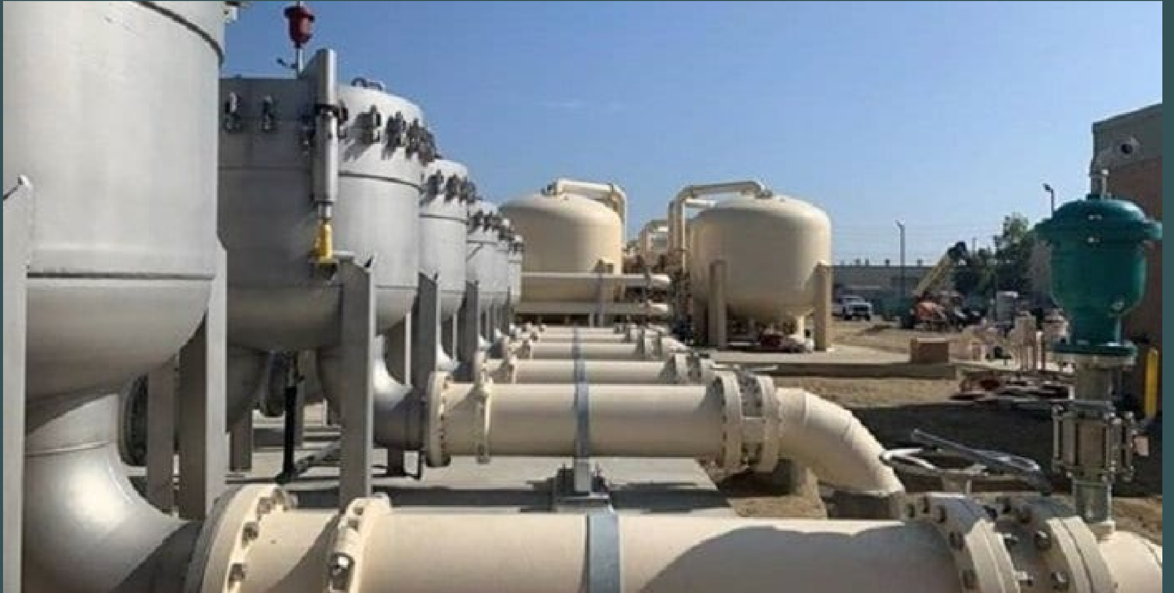
Orange County Water District & Yorba Linda Water District – U.S. largest IX treatment plant.
