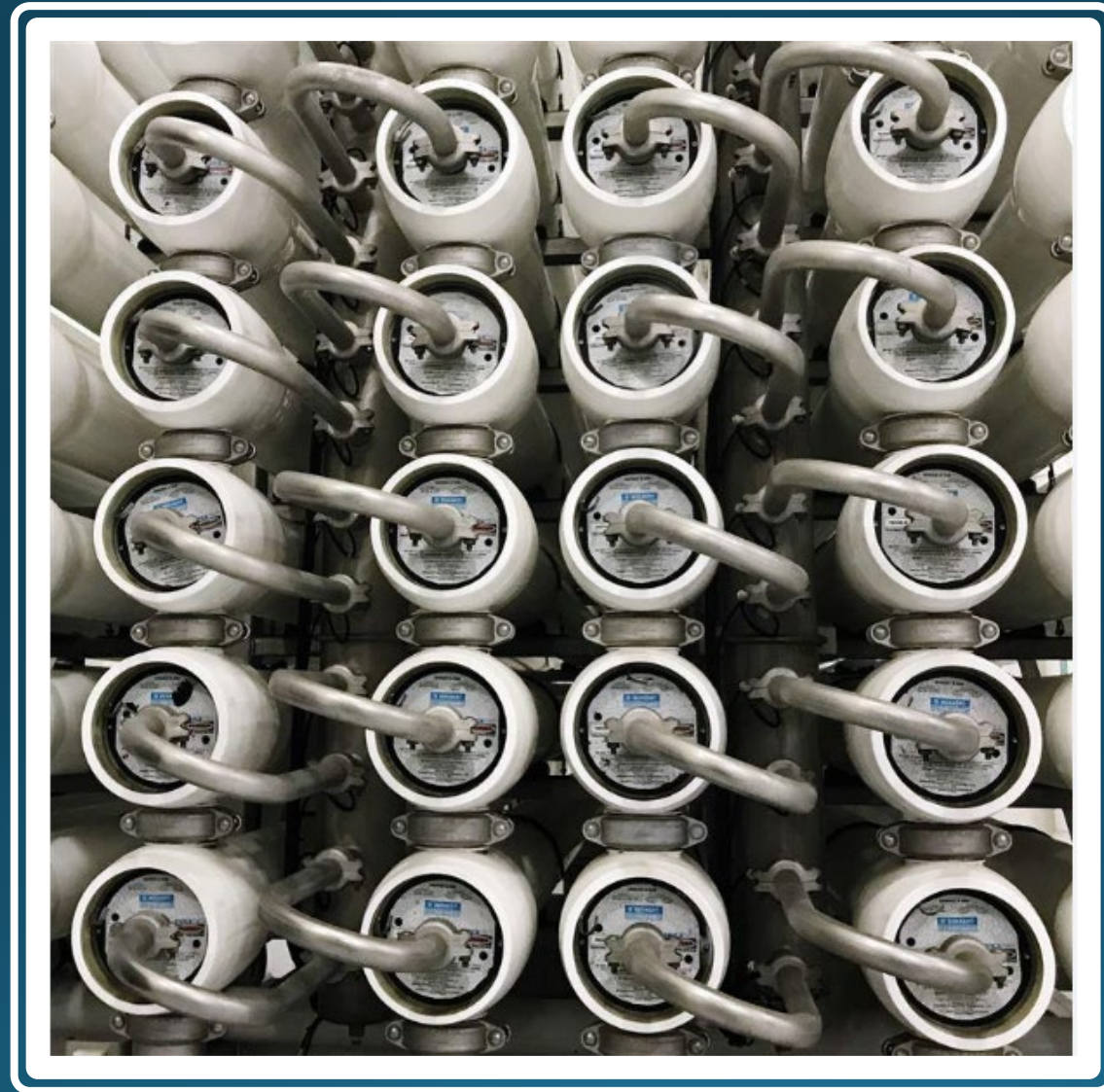
RO – Reverse Osmosis
