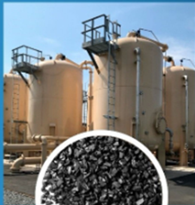
GAC - Granular Activated Carbon
