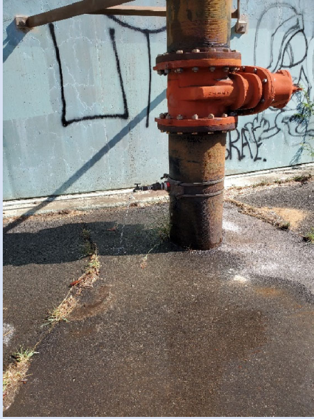
Site #7: Maui Lani Wells Chlorinator
