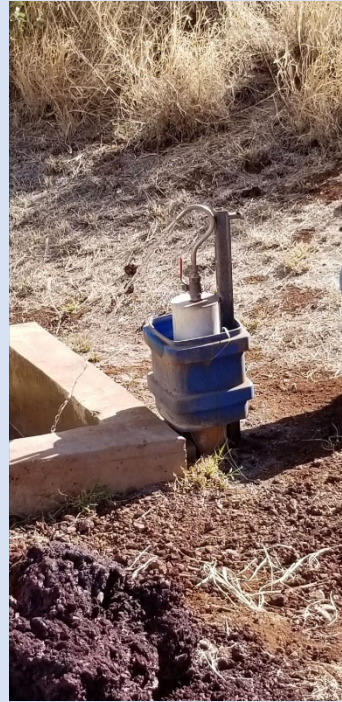
Site #13: Kawela Plantation Wells Chlorinator
