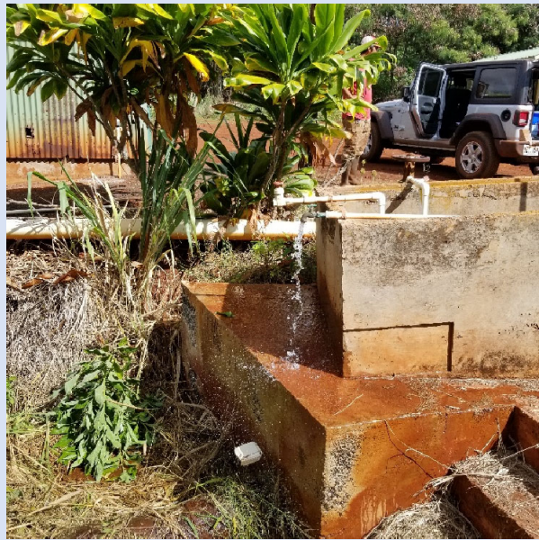
Site #11: Olokele Shaft Chlorinator
