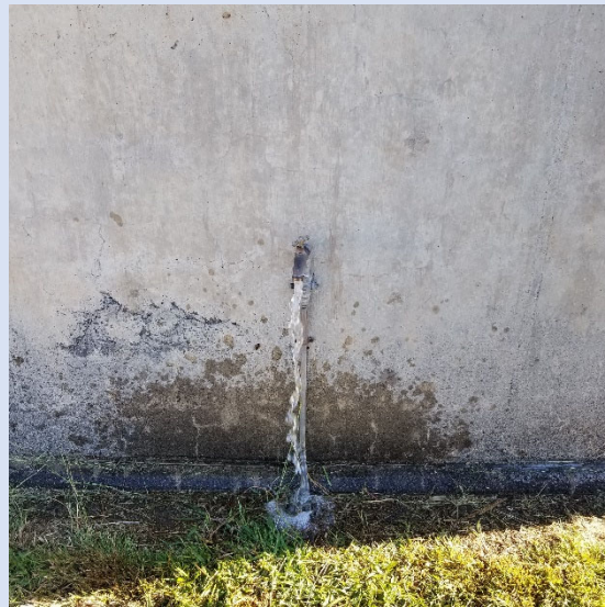
Site #12: Blend of Kauluwai Wells Chlorinator
