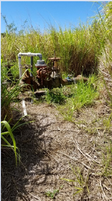
Site #4: Mokuleia Wells Chlorinator
