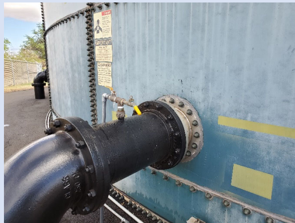
Site #8: Maui Highland Wells 1 and 2 Chlorinator
