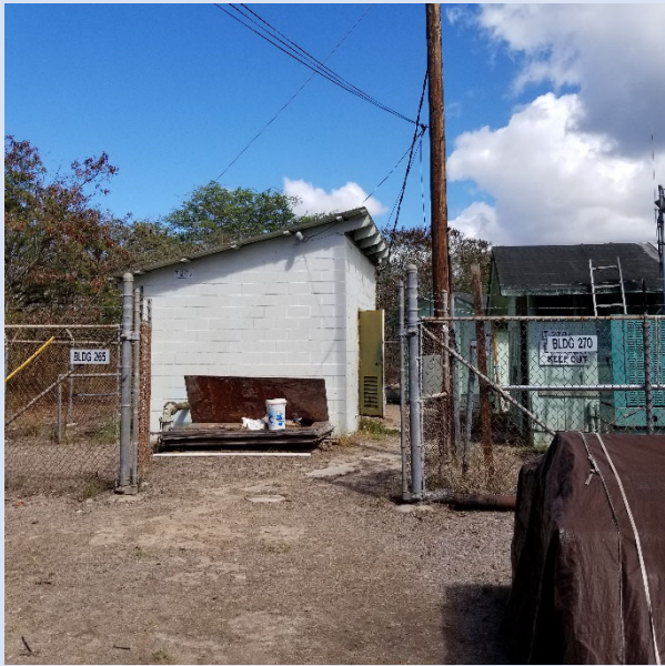
Site #5: Dillingham Well Chlorinator
