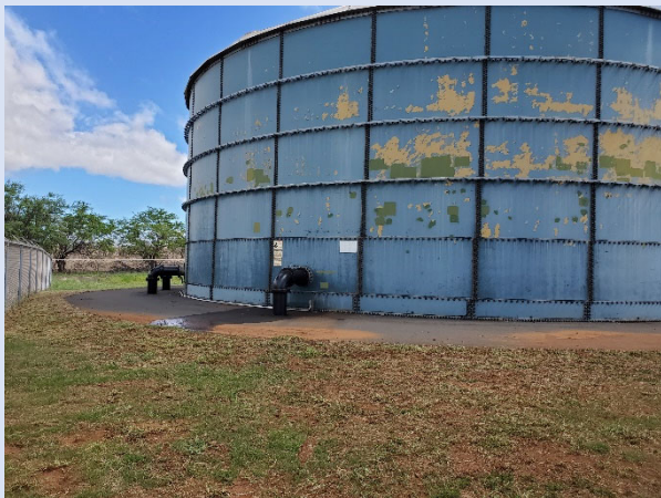
Site #8: Maui Highland Wells 1 and 2 Chlorinator
