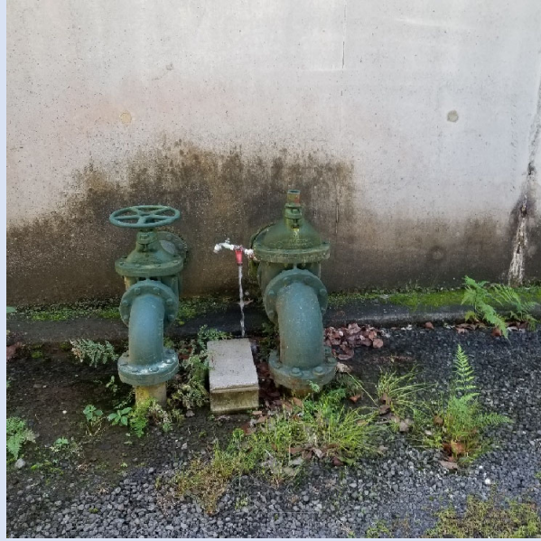
Site #19: Ookala Well Chlorinator
