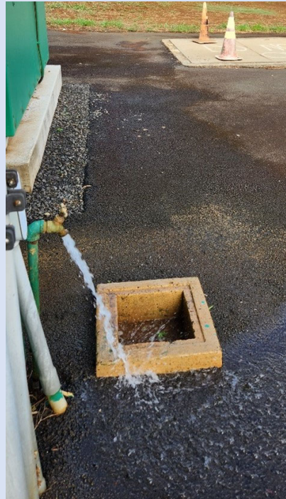
Site #10: Anahola Wells A, B and C Chlorinator
