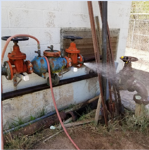
Site #5: Dillingham Well Chlorinator
