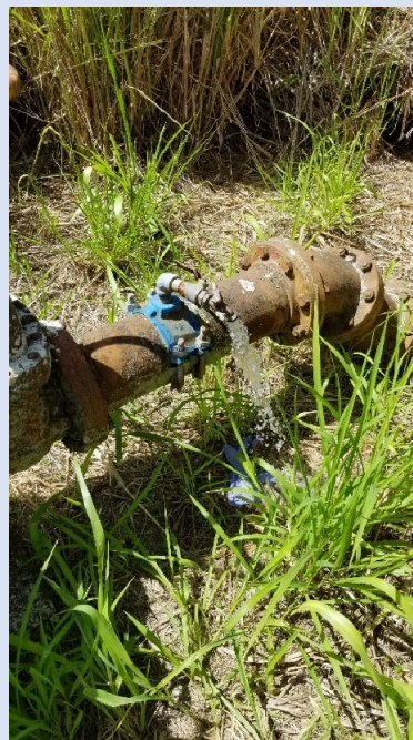
Site #4: Mokuleia Wells Chlorinator
