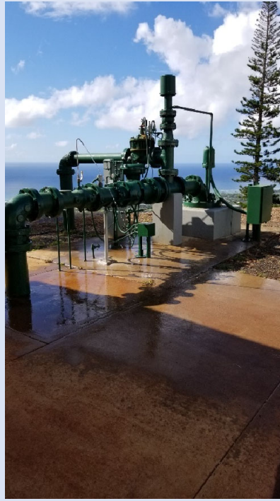
Site #1: Aina Koa Wells 2 Chlorinator
