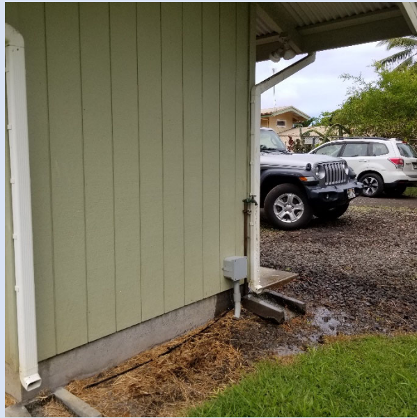
Site #21: Chaves Spring Chlorinator
