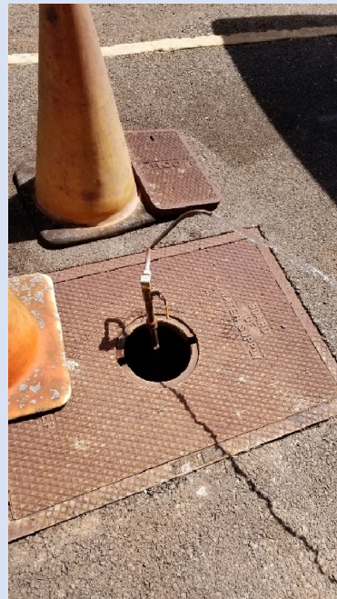
Site #2: Kahuku Wells Chlorinator
