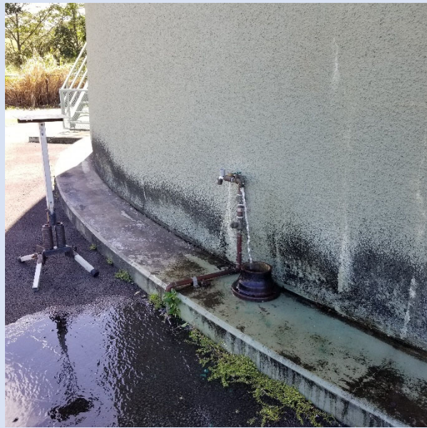
Site #20: Laupahoehoe Wells P1 and P2 Chlorinator
