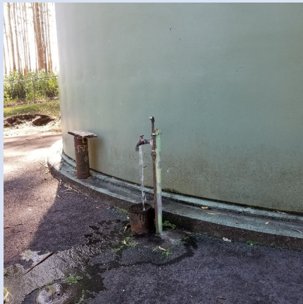
Site #18: Paauilo Well Chlorinator EPD
