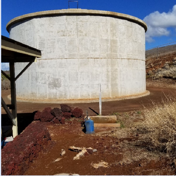
Site #13: Kawela Plantation Wells Chlorinator
