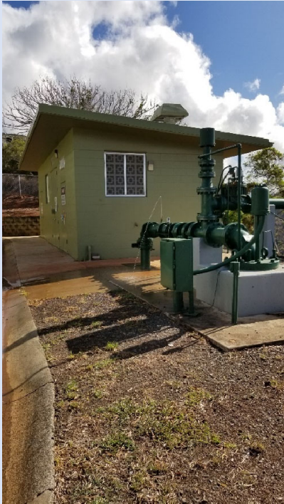
Site #1: Aina Koa Wells 2 Chlorinator
