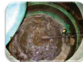
Figure 4. Aeration in an ATU.
