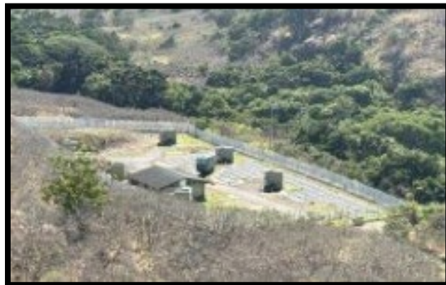
Solar Panels at a BWS well site ➤
