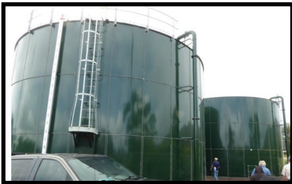
➤ New 228k-gallon steel tanks
