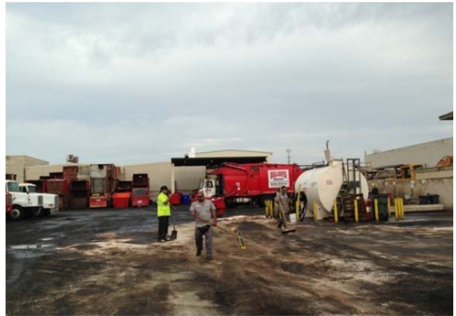
Roll-offs Hawaii Diesel Above Ground Storage Tank
