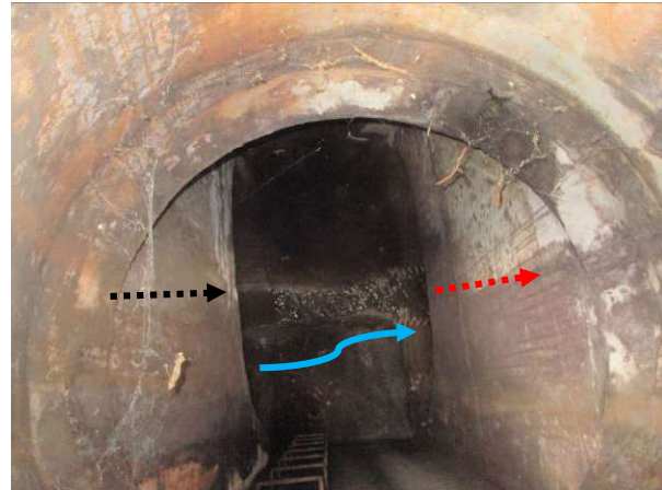
TMK: 9-4-128:002: View within the State Highways Division SDMH (PID 203145) of the dry weather flow with an alcohol odor discharging from a CCH 84-inch RCP (to the left) to a State Highways Division 84-inch CMP culvert (PID 700670) (to the right). (IMG_010)
