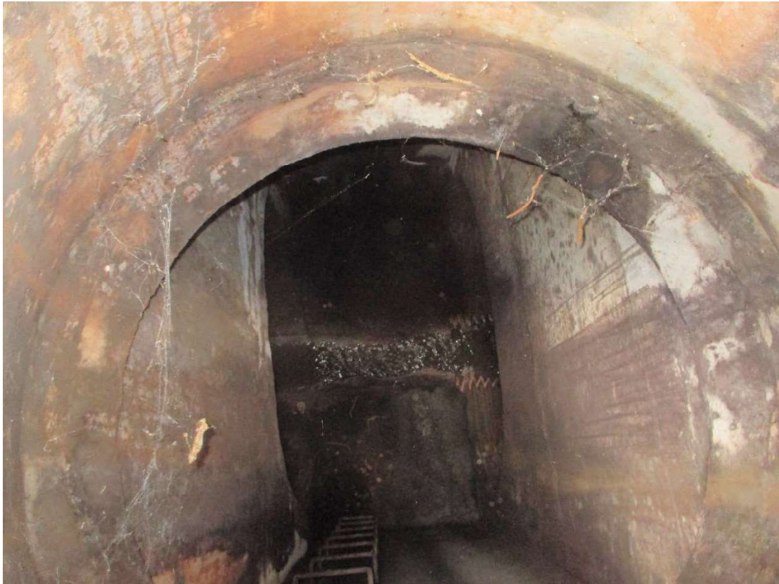
CCH 84-inch RCP (to the left) with dry weather flow with alcohol odor discharging to a State Highways Division 84-inch corrugated metal pipe (CMP) (to the right).
