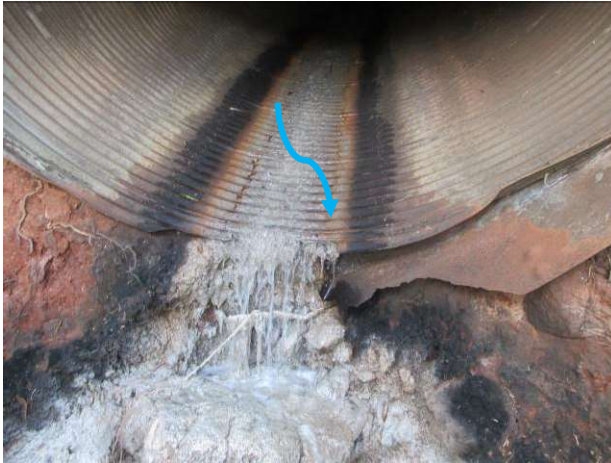
TMK: 9-4-128:002: Closer view of the State Highways Division outfall (PID 300732) with observed dry weather flow with an alcohol odor. Staining and mold observed within the outfall and covering the rocks surrounding the outfall. (IMG_005)
