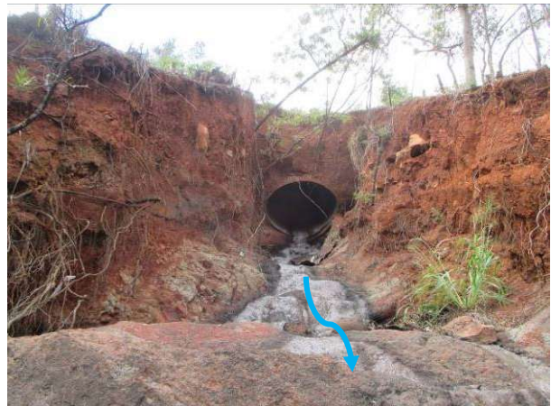
TMK: 9-4-128:002: State Highways Division outfall (PID 300732) along H-2 with observed dry weather flow with an alcohol odor. Staining and mold cover the rocks surrounding the outfall. (IMG_004)
