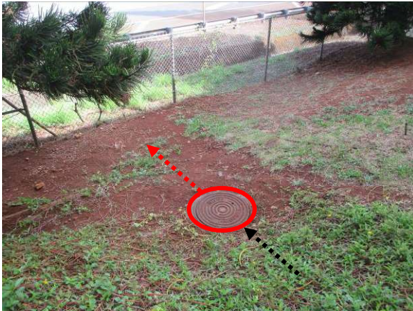
TMK: 9-4-128:002: State Highways Division storm drain manhole (SDMH) (PID 203145) located near the southeastern perimeter of the property with access to the CCH 84-inch RCP and a State Highways Division 84-inch corrugated metal pipe (CMP) culvert (PID 700670). (IMG_009)
