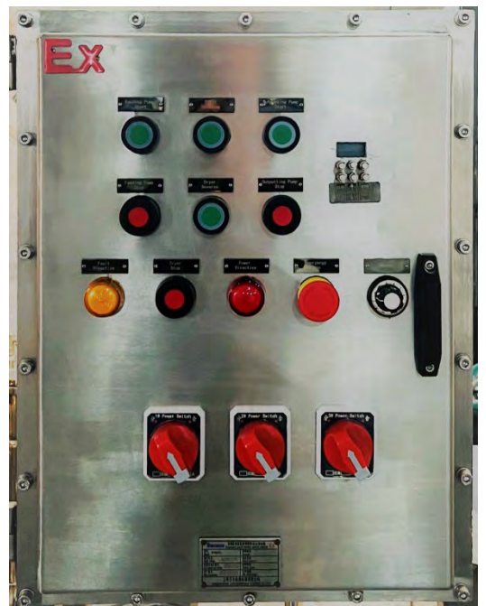
Control box on Extraction Skid
