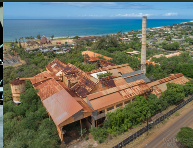
Insufficient Processing Plant
