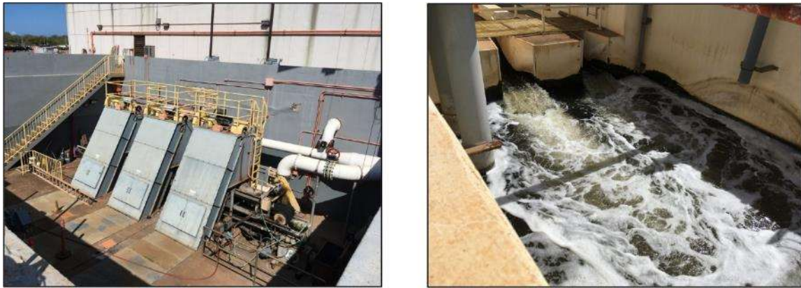
Figure 1. Influent intake and effluent discharge culvert at a WWTP. Effluent discharges to ocean.
