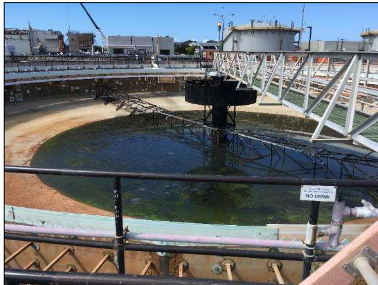
Figure 2. Wastewater treatment plant clarifier used for settling and collection of biosolids from wastewater influent.
