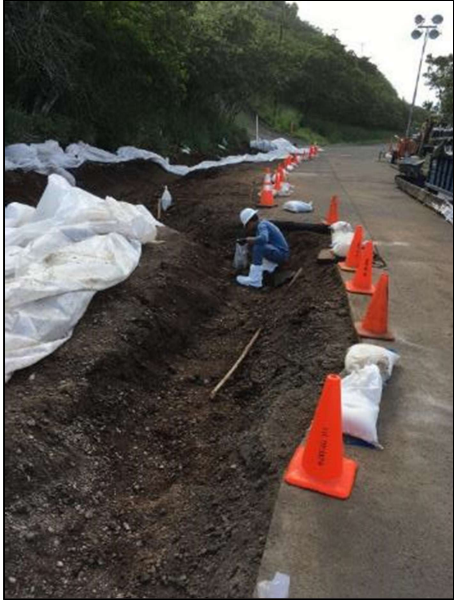
Figure 5. Excavation trench designated as a Source Area Decision Unit for collection of a single, Multi Increment sample. Used to confirm cleanup of an AFFF release.
