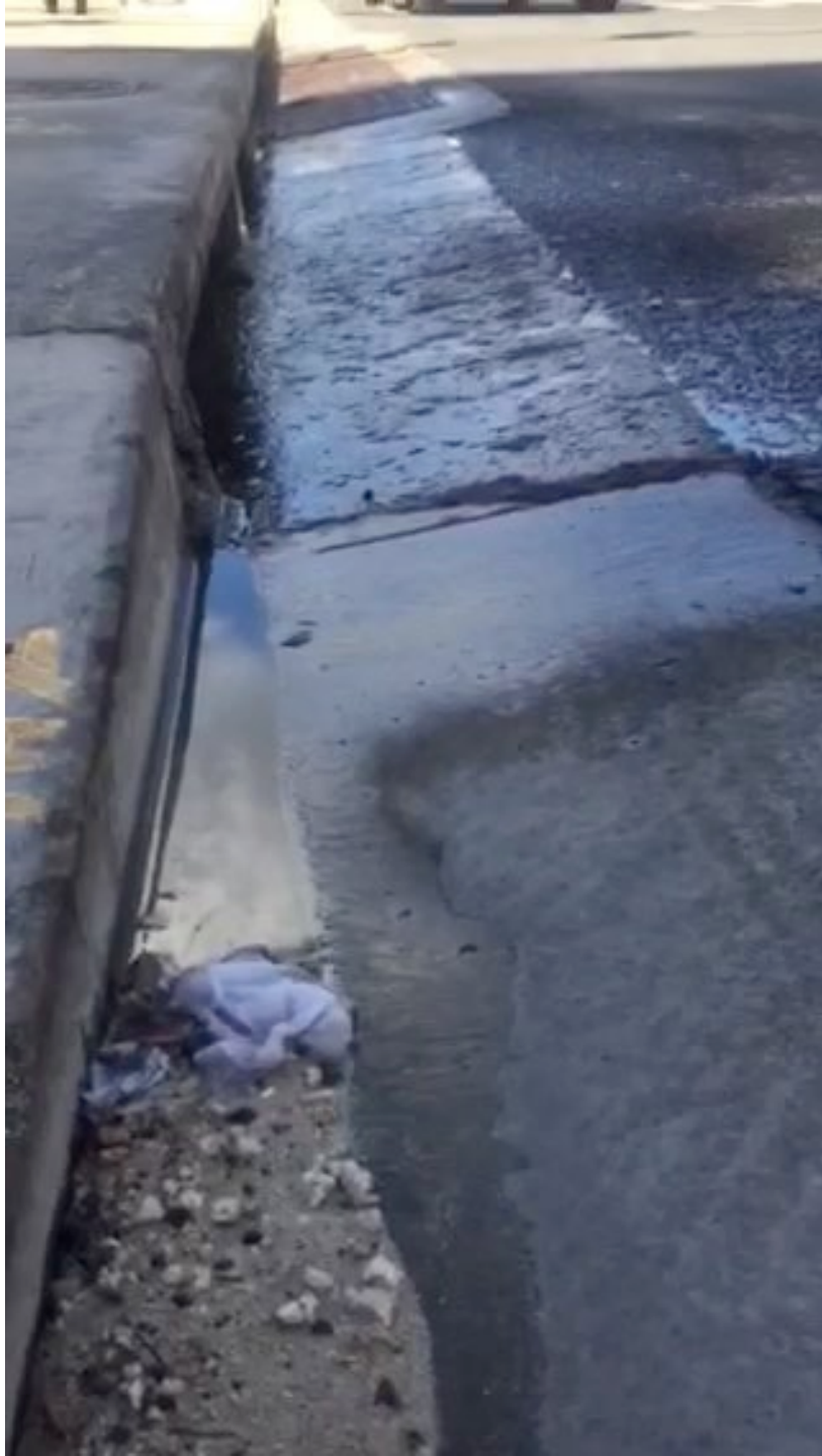
Storm drain backflow
