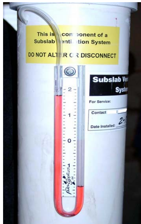
Figure 5.1 Manometer indicating the SSD system is operating properly.
