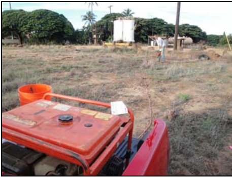
c) Use of hi-powered, Hilti drill with a portable generator (photo from Weston Solutions).
