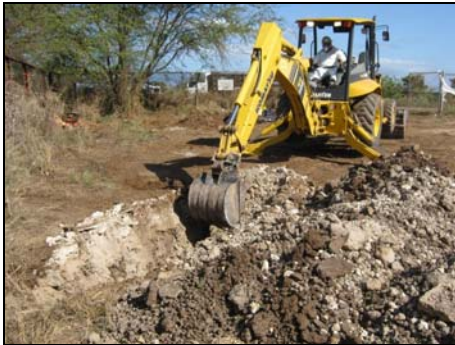
i) Trenches and potholes for soils within a few feet of the ground surface (photo by EnviroServices & Training Center, LLC).
