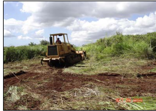
b) Bulldozer used to cut access path into to one of fifty-nine, lot-size DUs within several thousand acre field (photo from Bureau Veritas).
