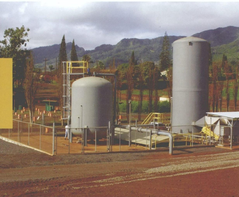
Groundwater treatment system at the Del Monte Superfund site, Kunia, Hawaii.
