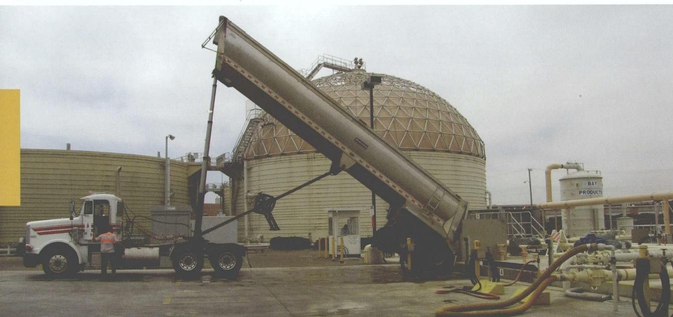
A truck offloads food waste on its way to EBMUD’s dome-shaped anaerobic digester.
