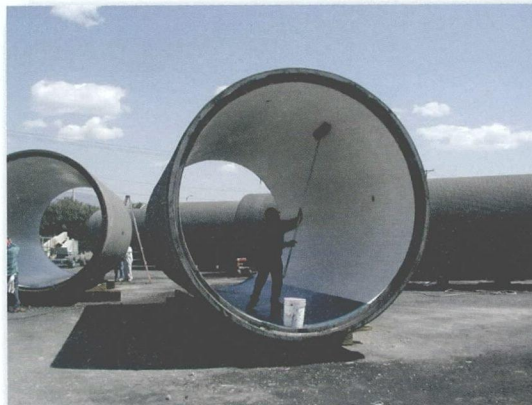
Preparing sections of new sewer pipe — part of Los Angeles' effort to curb sewage spills.
