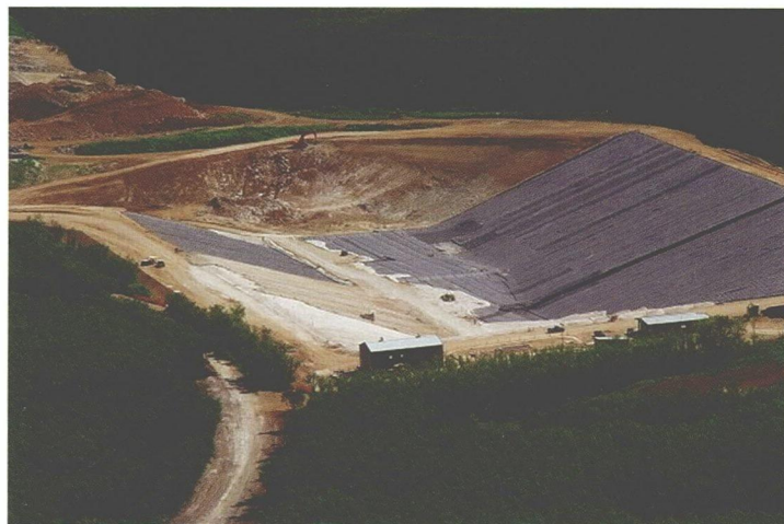
Saipan's new Marpi Landfill under construction. The new solid waste landfill, first in the Pacific Islands to comply with federal standards for preventing pollution, opened in February 2003.
