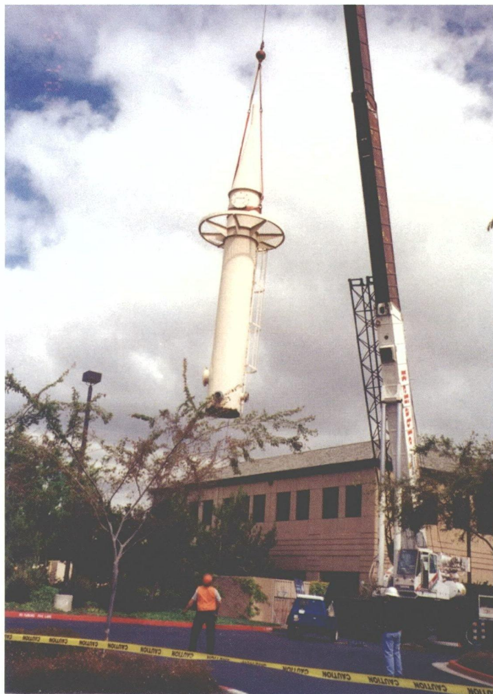
In Mountain View, Calif., responsible parties removed equipment that had treated TCE-contaminated groundwater by air-stripping, and replaced it with systems that release no TCE into the air.
