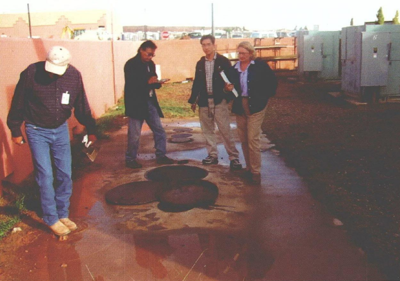
Navajo Nation EPA and U.S. EPA staff inspecting an underground fuel storage tank facility at Chinle, Navajo Nation. In 2003, EPA's underground storage tank program trained many tribal UST inspectors.
