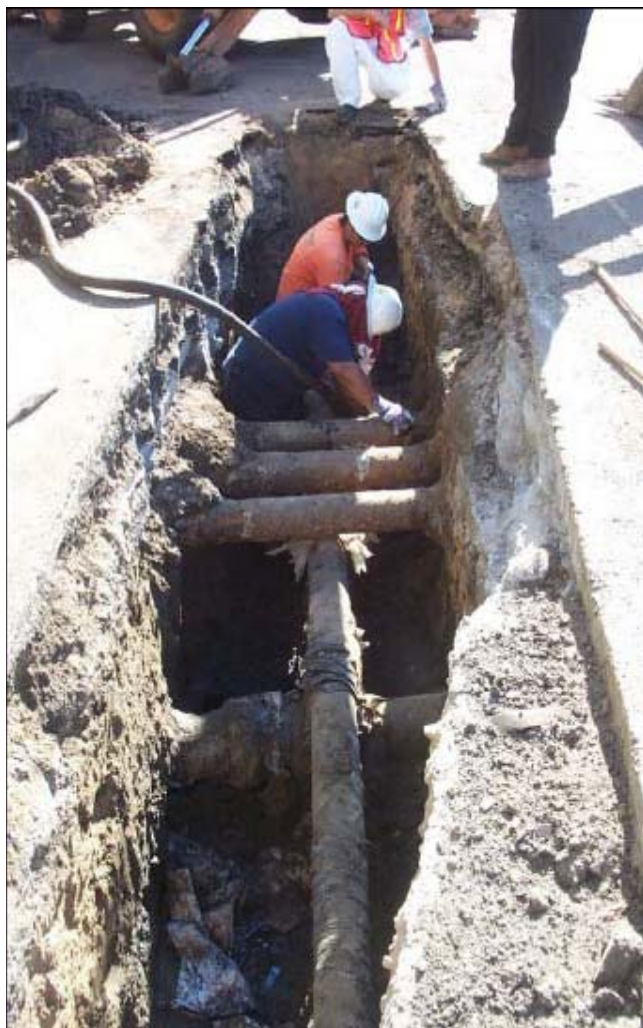
Honolulu Harbor Iwilei District Pipelines in HECO Trench Near Flora Dec
