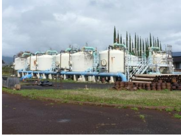
Photo 12d: Granular Activated Carbon
