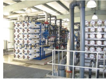
Photo 12f: Reverse Osmosis
