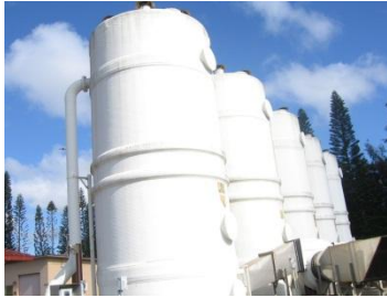
Photo12e: Packed Tower Aeration
