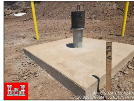
Figure 3. Groundwater monitoring well MW-02.
