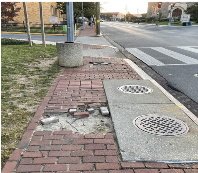
Figure 17: Example of deteriorated brick sidewalk
