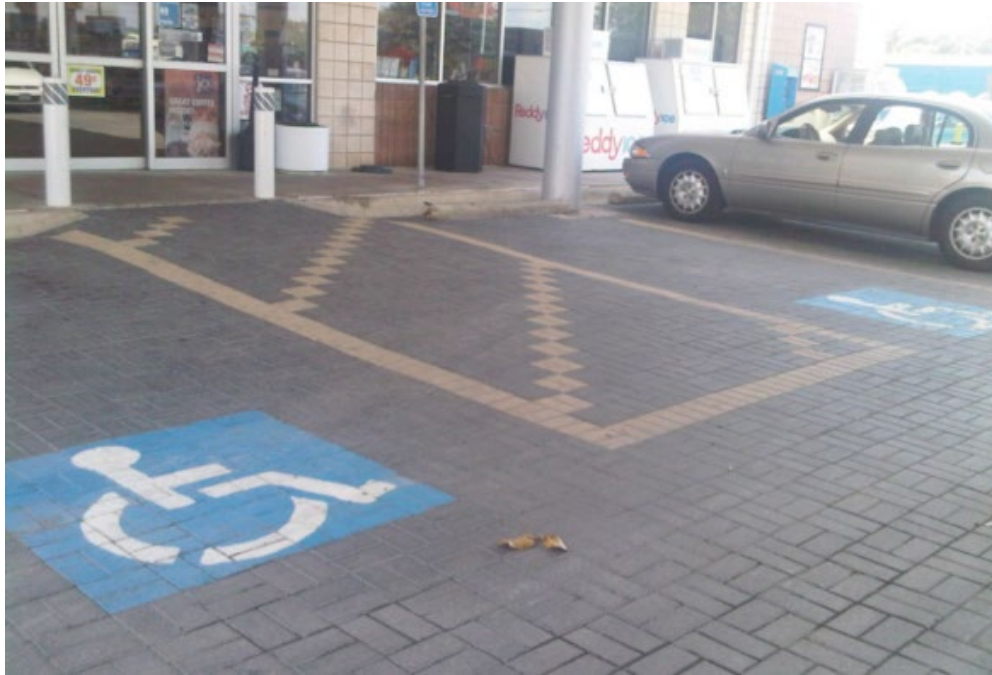
(Visible slope in parking spaces and access aisle)
