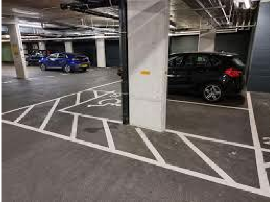
(Pillar impedes access)
