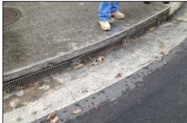
The City MS4 in Wahiawā has filters at some of the stormwater inlets to prevent debris and other pollutants from entering the system
