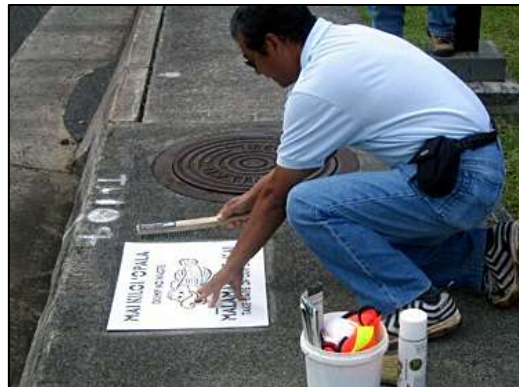
Stenciling at storm drain inlets informs the public not to dump anything down the drain
