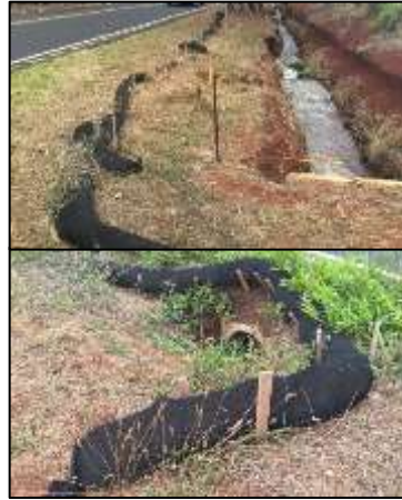
These barriers ("bio-socks") are a temporary BMP placed along Kaukonahua Road help prevent the transport of sediments and other pollutants that are common in runoff from roadways
