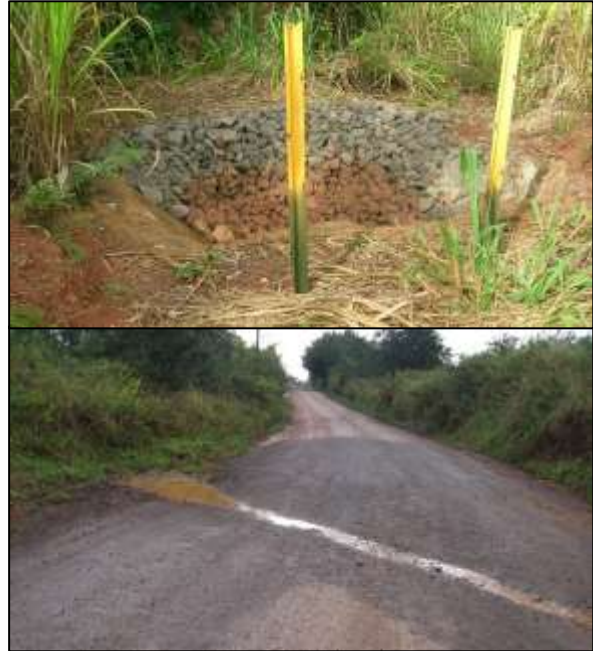
Two examples of practices implemented in Schofield Barracks East Range: Sediment pit (top); Broad-based dip for channeling and directing stormwater (bottom)
