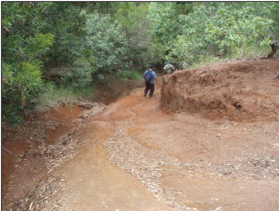
Photo B26: View of erosion by surface runoff from bedrock exposure at lookout in Kolekole Pass.
