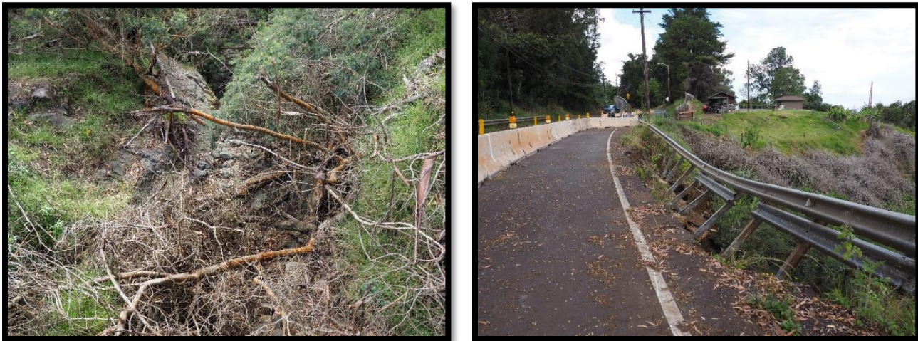
Figure 52. Clogged Drainage Infrastructure and Flooding Impacts on Roadways
