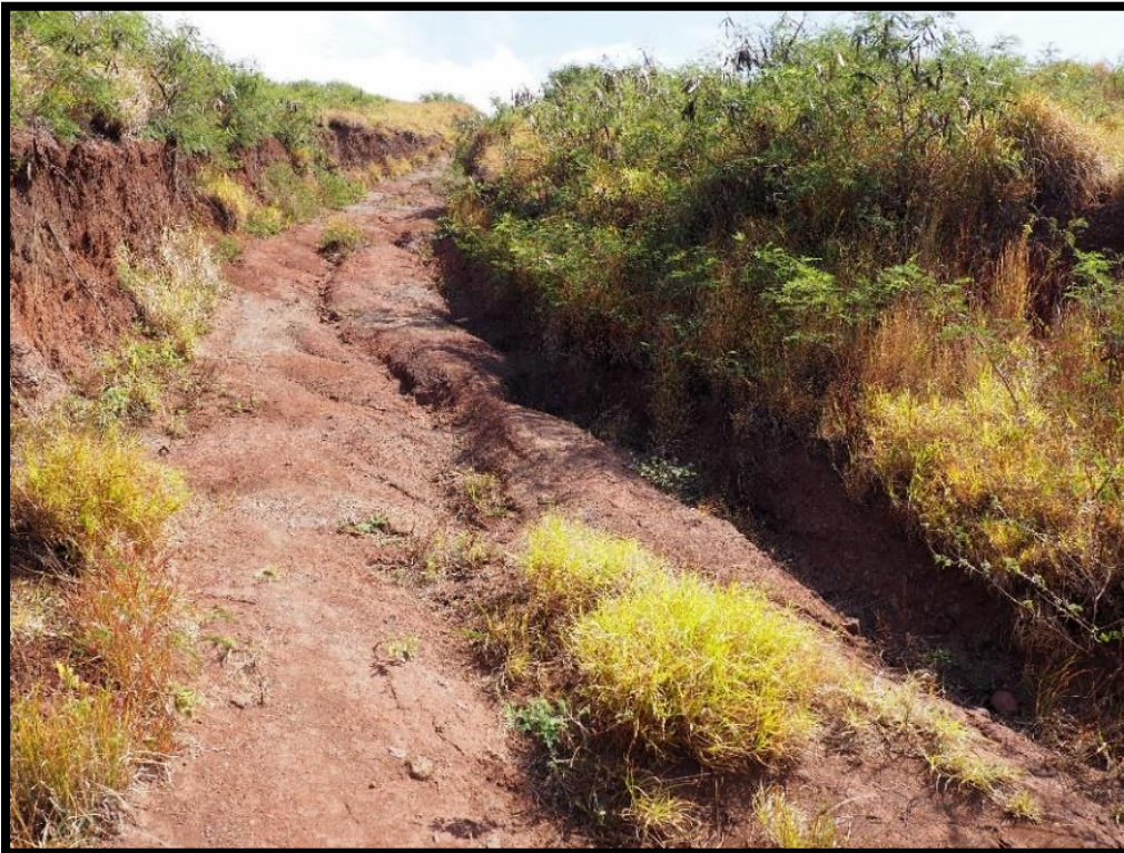
Figure 47. Example of Unmaintained Dirt Road
