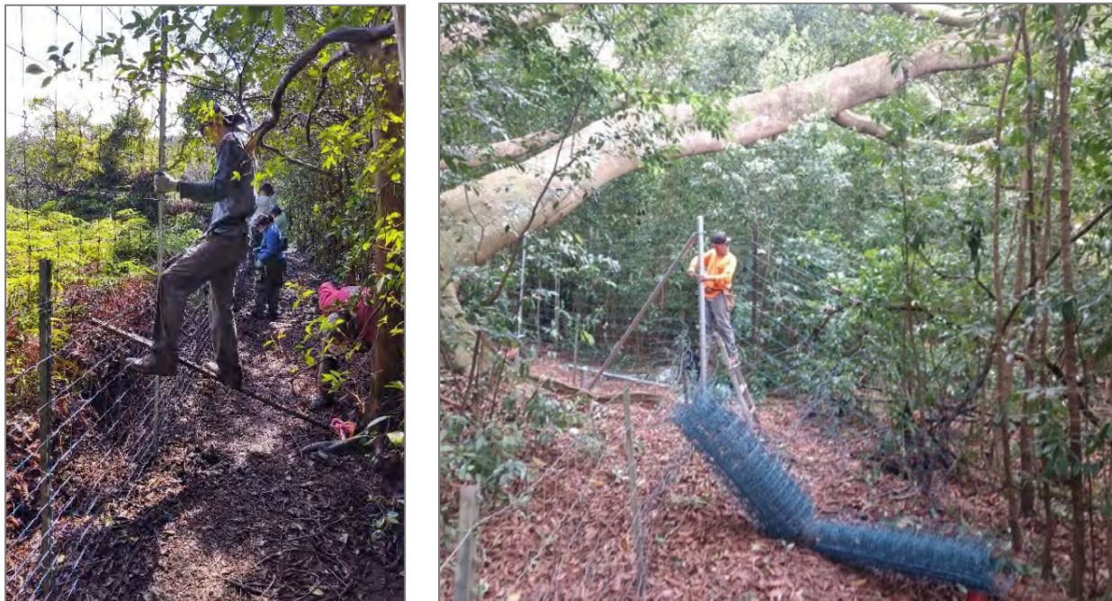
Figure 8. Ungulate exclusion fence being retrofitted and improved (left) and installed (right) as part of the Section 319-funded "Polluted Runoff Control Project for West Maui" (2018-2022) being implemented by the Department of Land and Natural Resources, Division of Forestry and Wildlife
