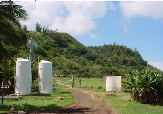
The reactors (two anaerobic on the left, one aerobic on the right) collect animal wastewater/milking parlor wastewater, provide highly efficient treatment, and allows the water to be reusable for irrigation or flushing.
