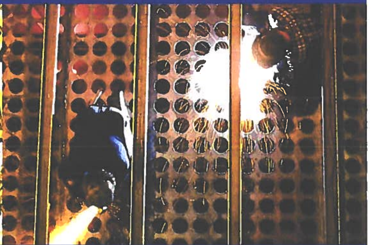
The tube sheet separates the dirty and clean air plenums. The dirty air must pass through the bags.
