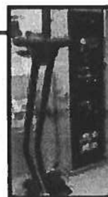
Upper Control Panel
