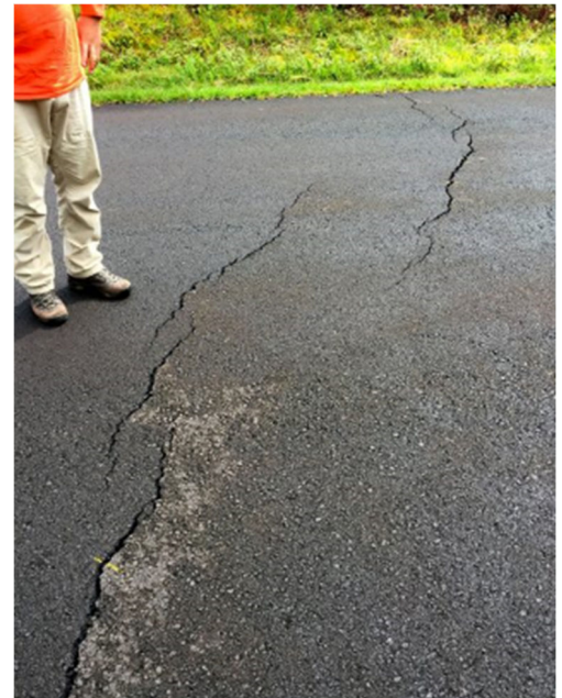
Cracks in road around Leilani Estates. Photo taken on 5/2/2018 courtesy of USGS.
