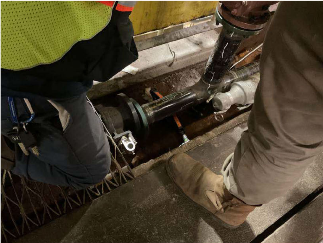
Ball valve installed downstream allowing simultaneous tank bottom draining via FOR line and groundwater through the Sump.
