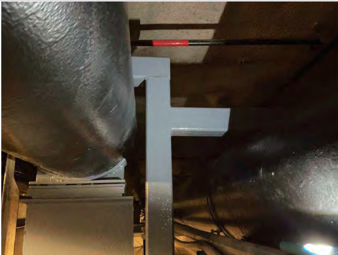
New welded bracket and saddle at Pipe Support 74. Horizontal member prevents "escape" of F-24 line.
