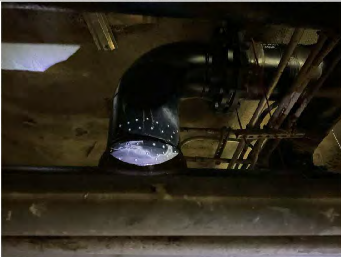
18x12 branch connection by welded o-let connection. Array decals from PAUT examination.
