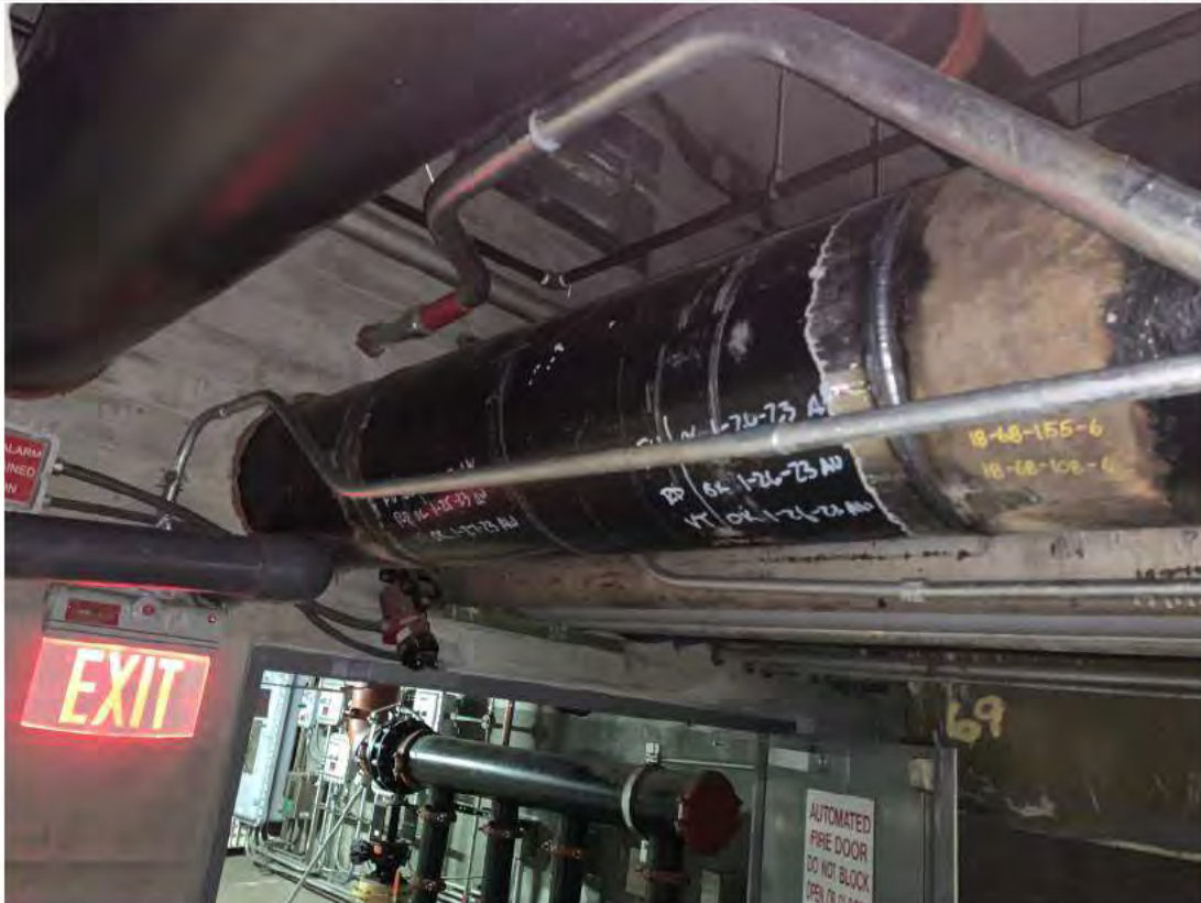
Downhill side of the Door 3 bulkhead penetration between PS 68 and 69; no existing photograph of bell connection available.
