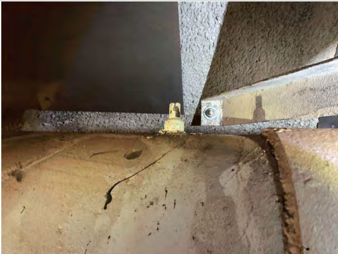
Seal welded assembly at PS 312; no repair performed.
