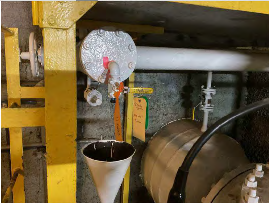
New threaded plug installed on (b) (3) (A) nipple on FOR line at Surge Tank 4.
