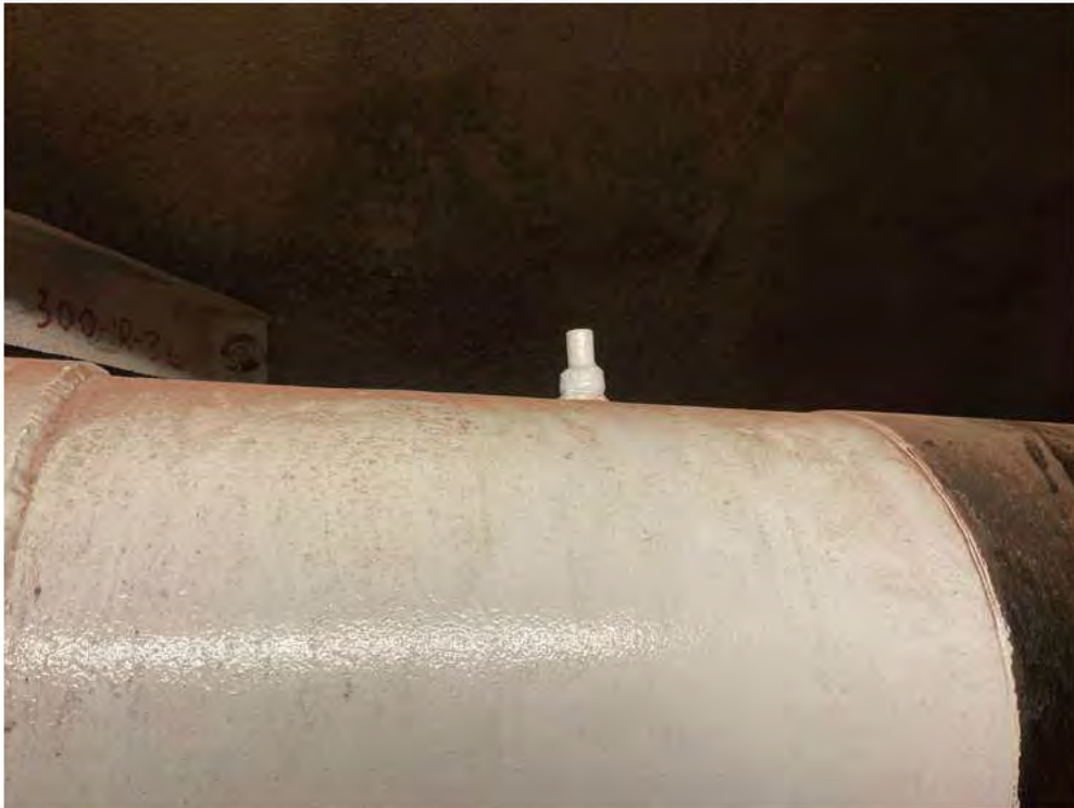
Existing plug at PS 144 seal welded; no repair performed.
