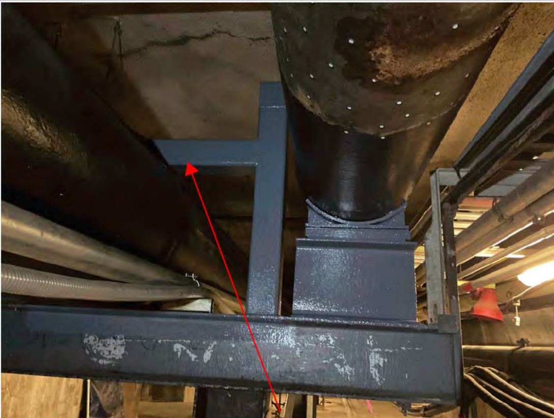
New welded bracket to prevent "escape" of JP-5 line at existing Pipe Support 74.
