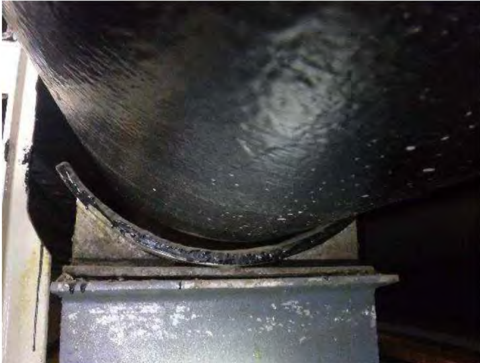
Representative photo of existing conditions within Pipe Support range.
