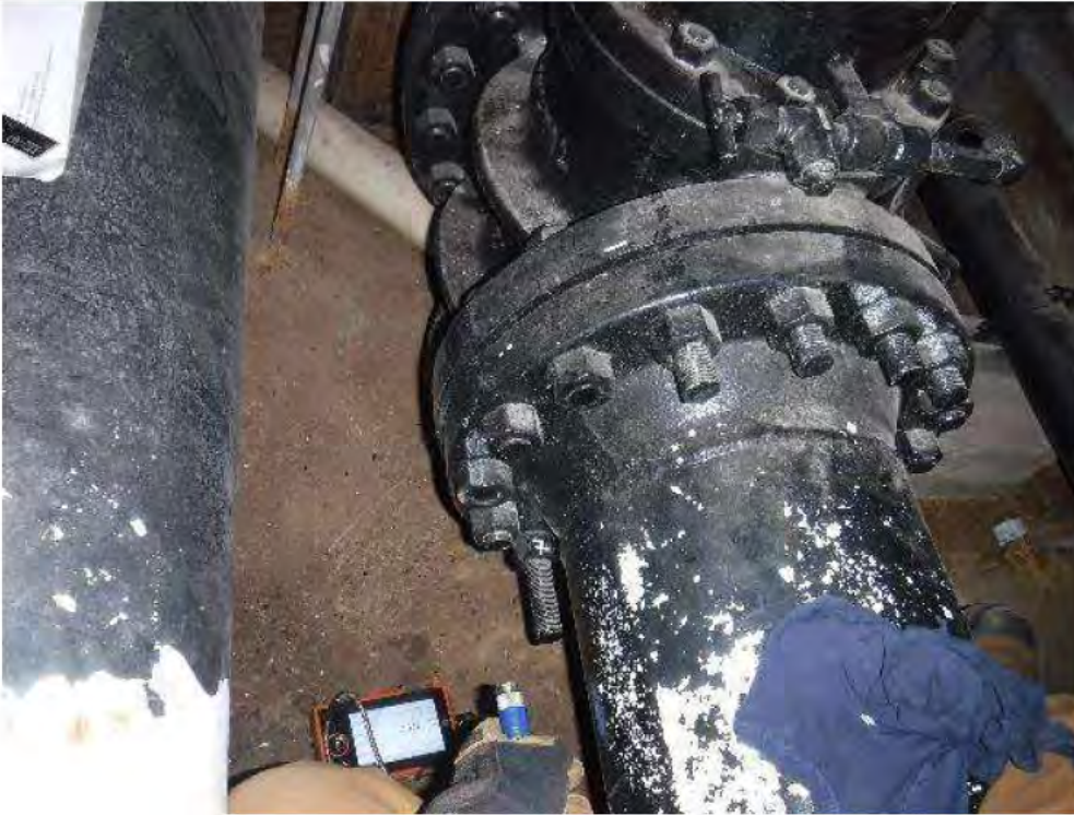
Existing fasteners at 16-inch flange not properly sized.
