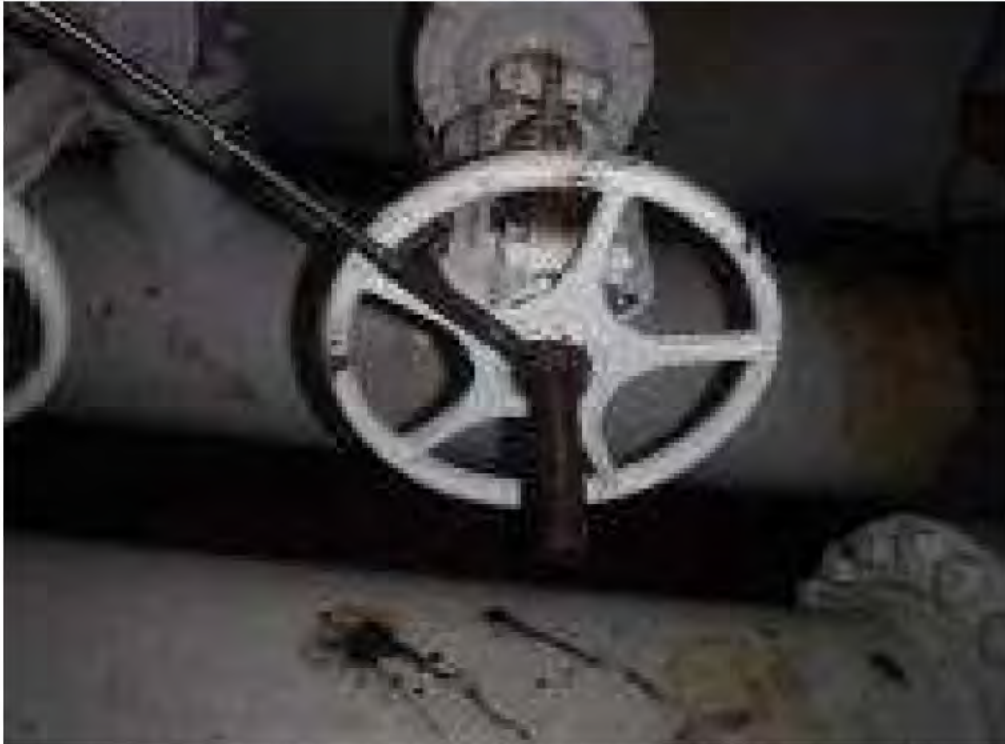
Existing condition: valve handwheel missing thread nut. Note: valve in open position in photograph.
