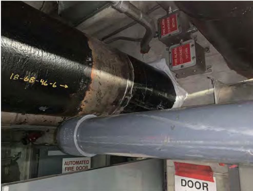
Uphill side of the Door 3 bulkhead penetration between PS 68 and 69; no existing photograph of bell connection available.
