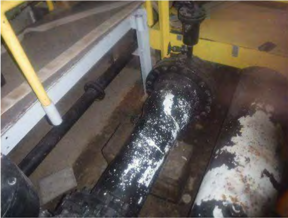
Existing threaded high point vent assembly at UGPH bulkhead.
