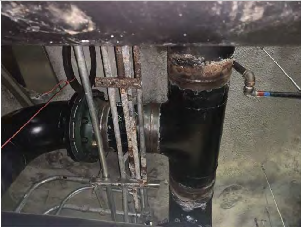
Branch connection to tank lateral piping. No existing condition photograph available.
