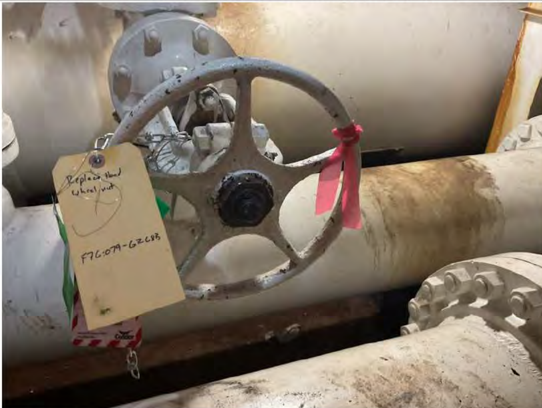
Contractor installed nut on handwheel. Note: valve in closed position in photograph.
