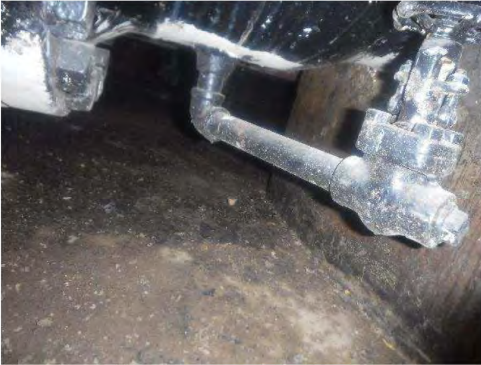
Existing threaded low point drain assembly at UGPH bulkhead.
