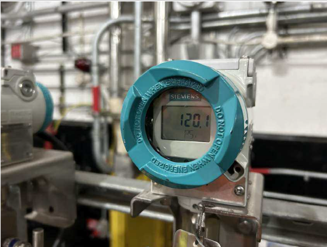
Line segment tested with Nitrogen at 120 psi for 1 hour, with soap testing at affected joints. No leaks noted.
