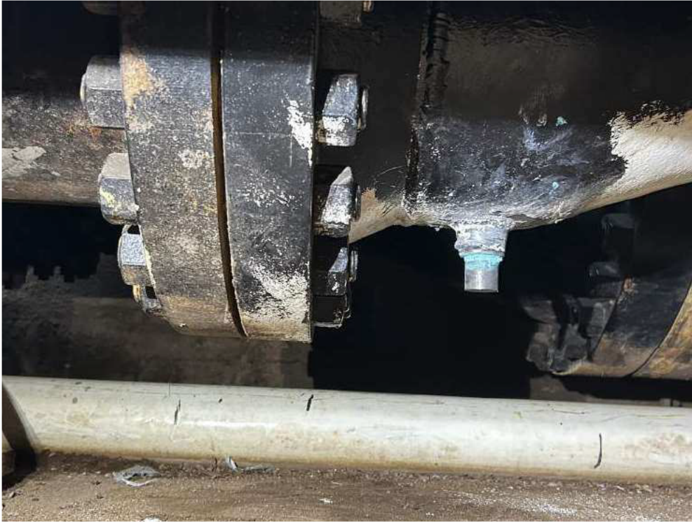
Low point drain assembly replaced with threaded plug after draining segment, cleaning threads and applying sealant.
