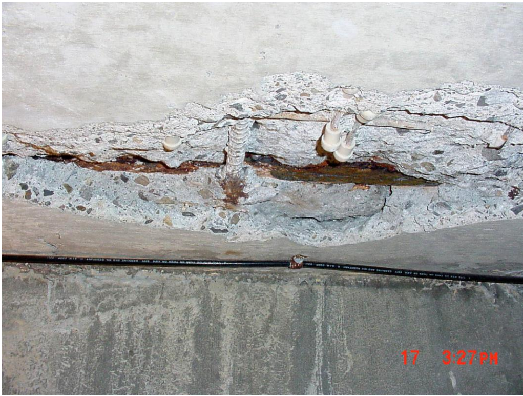
Figure 7-4 – Typical Exposed Reinforcement at Spall (Not from Subject Site)
