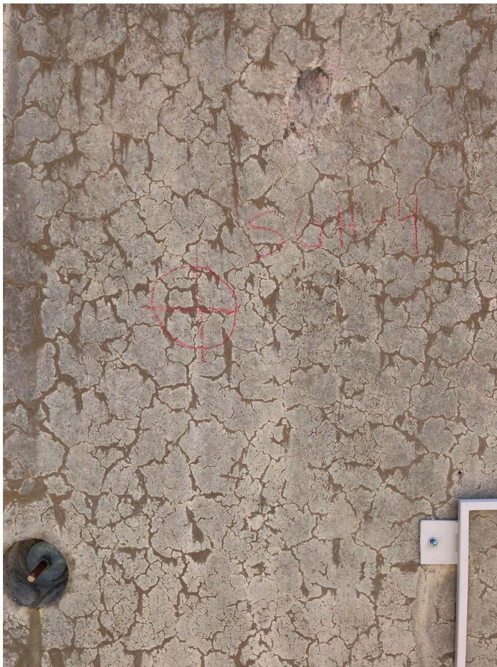
Figure 7-1 – Typical ASR Cracking (Not from Subject Site)
