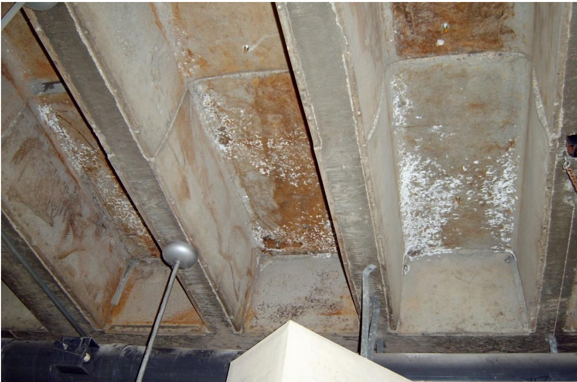
Figure 7-3 – Rust-Colored Staining (Not from Subject Site)
