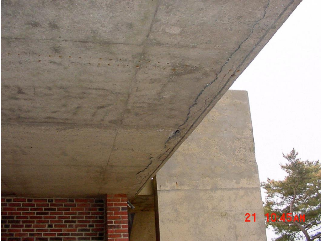
Figure 7-2 – Typical Incipient Spall (Not from Subject Site)
