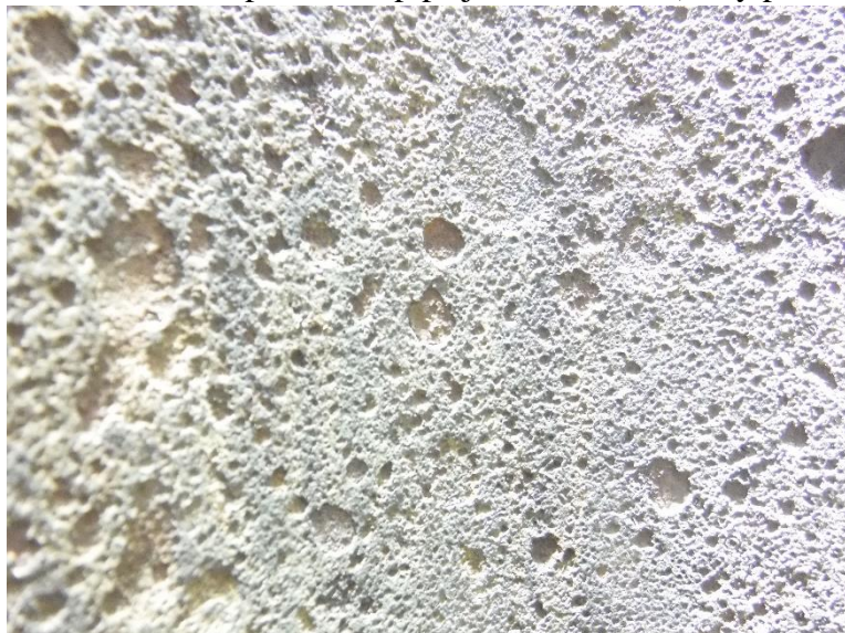
C.6 Close up of internal pitting just below tee
