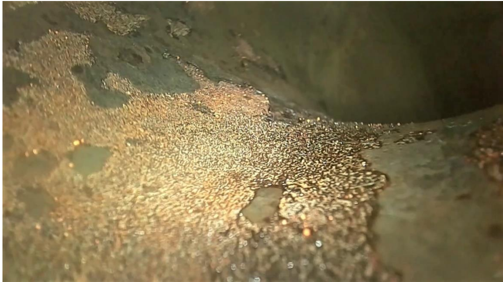
C.14 Second elbow 6 o'clock (minor erosion corrosion on inner radius) (from entry point A)
