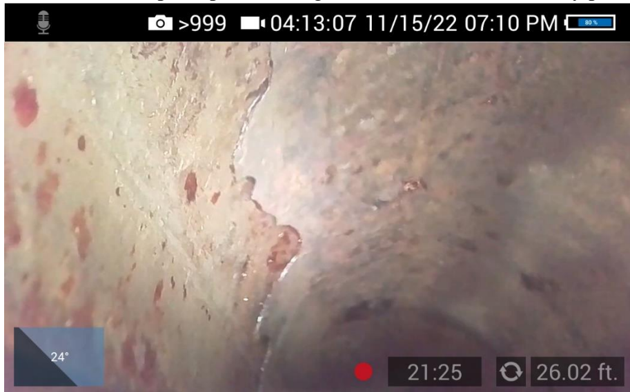
C.35 Borescope inspection image, ERW joint and mill scale (from entry point B)
