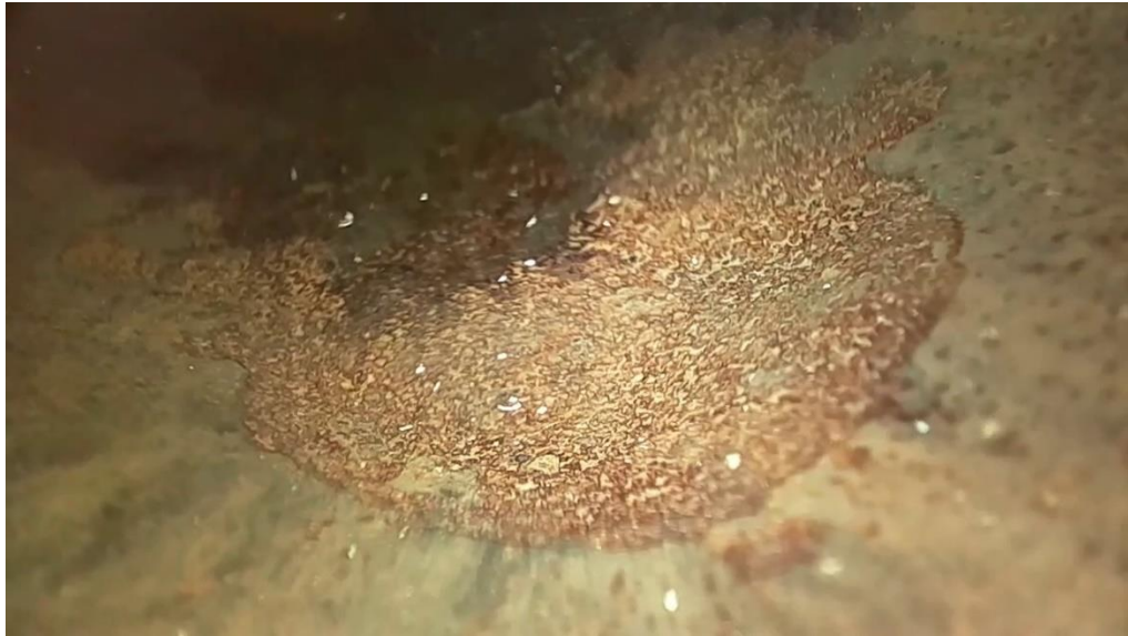
C.10 Borescope inspection image of 1st elbow erosion (from entry point A)
