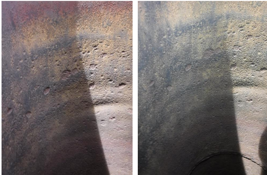
C.5 Interior portion of pipe just below tee (entry point A)
