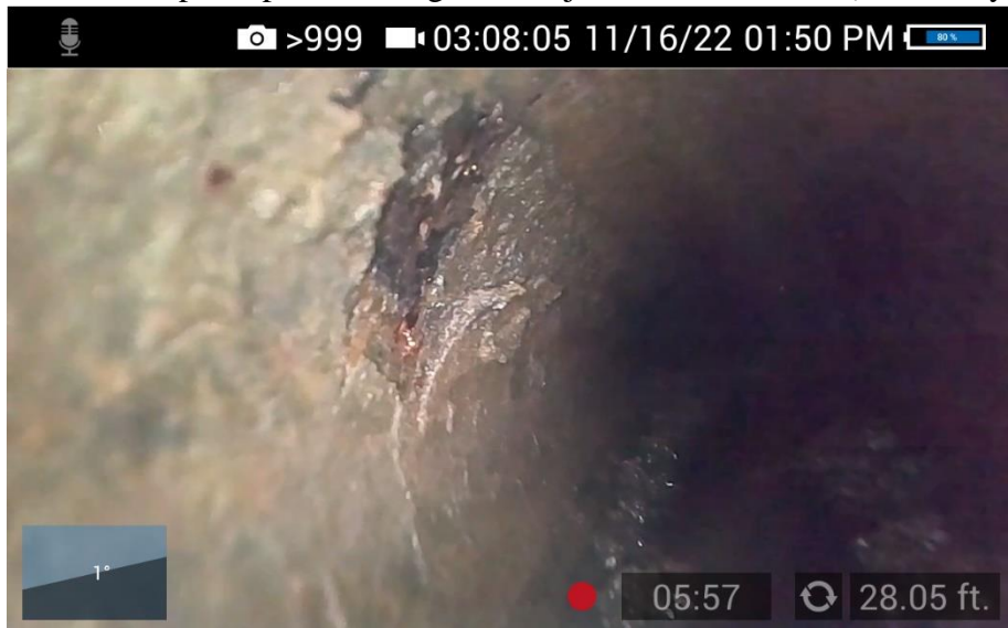
C.36 Borescope inspection image, mill scale (from entry point B)
