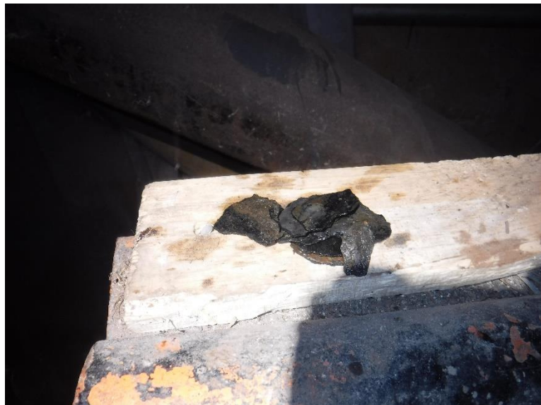
C.24 Entry Flange B (Scale and debris removed from pipe)
