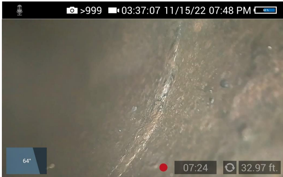
C.34 Borescope inspection image, 3 rd elbow weld (from entry point B)
