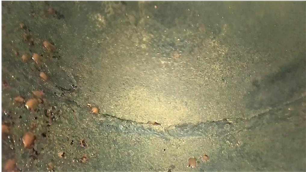
C.13 Second Elbow weld 10 – 1 o'clock (from entry point A)
