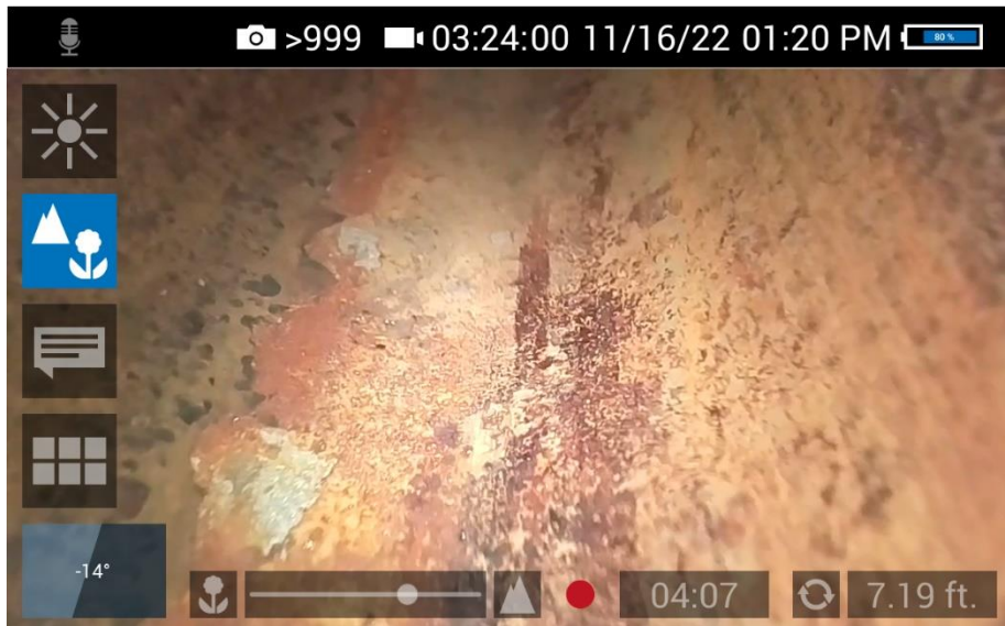
C.33 Boreoscope inspection image, bottom of pipe (from entry point B)
