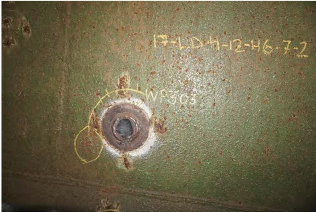
Photo 20: Poor welds at existing repairs on lower dome
