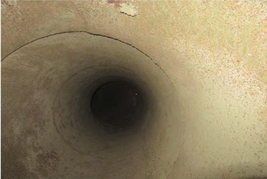
Photo 5: Vent piping at upper dome near upper access manway
