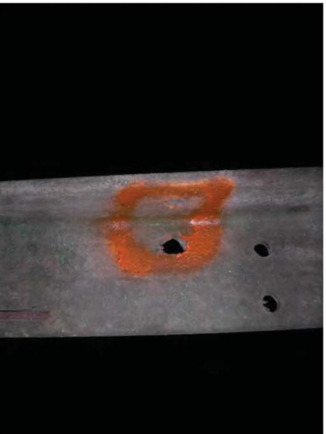
Photo 11: Tank #17 framing – Holes need patching with steel plate
