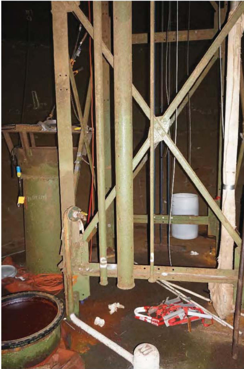
Photo 22: Abandoned stilling well and counterweight tubes at tank floor
