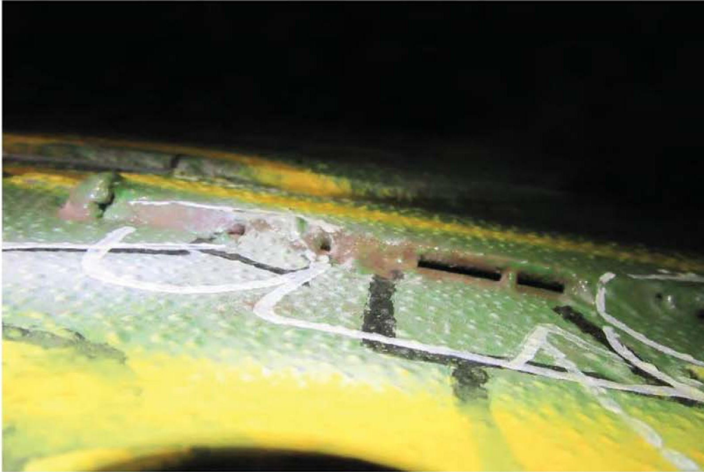
Photo 13: Backing bar not welded to plate
