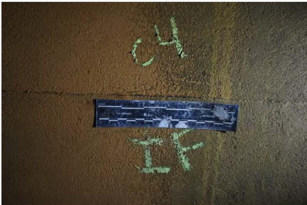
Photo 26: Insufficient fill in circumference weld of 32-inch line
