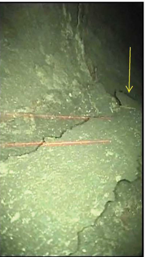
Photo 1: Large flake of corrosion product, several inches long.
