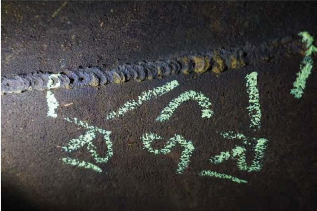
Photo 27: Rounded indications in Circumference Weld 5 of 32-inch line
