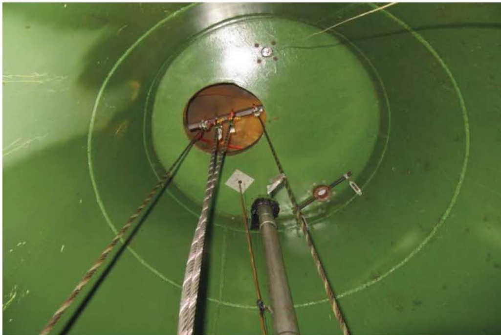
Photo 4: Upper access manway with ATG
