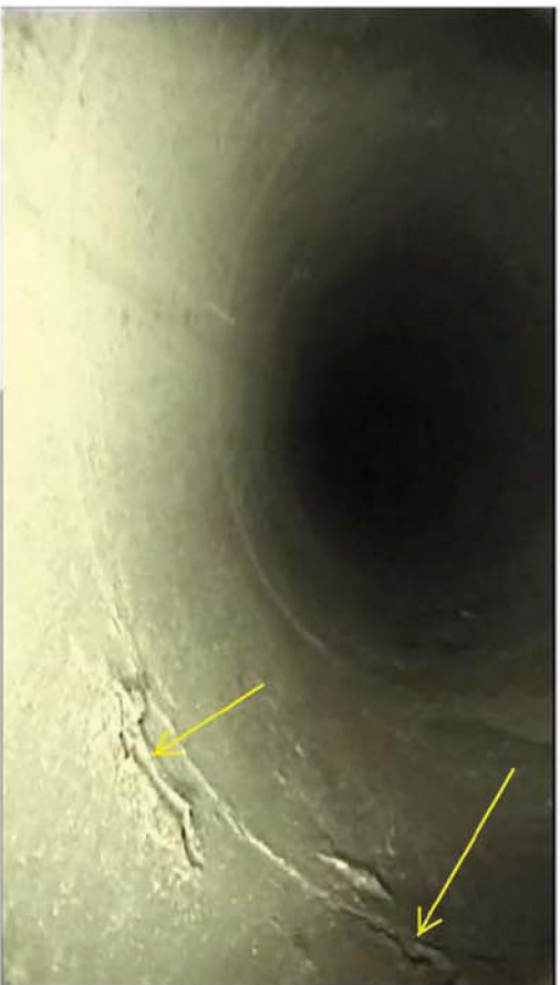
Photo 4: Holes and rust along spiral weld.
