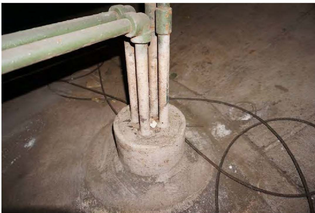
Photo 21: Sampling lines' tank floor penetration.
