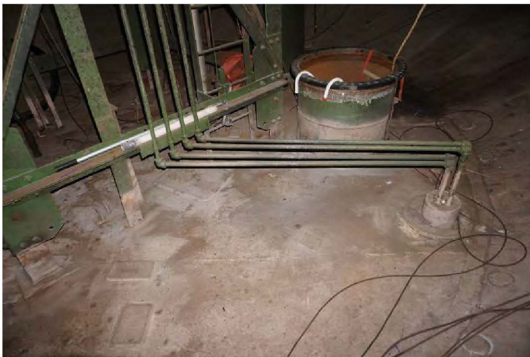
Photo 20: Sampling lines at tank floor.
