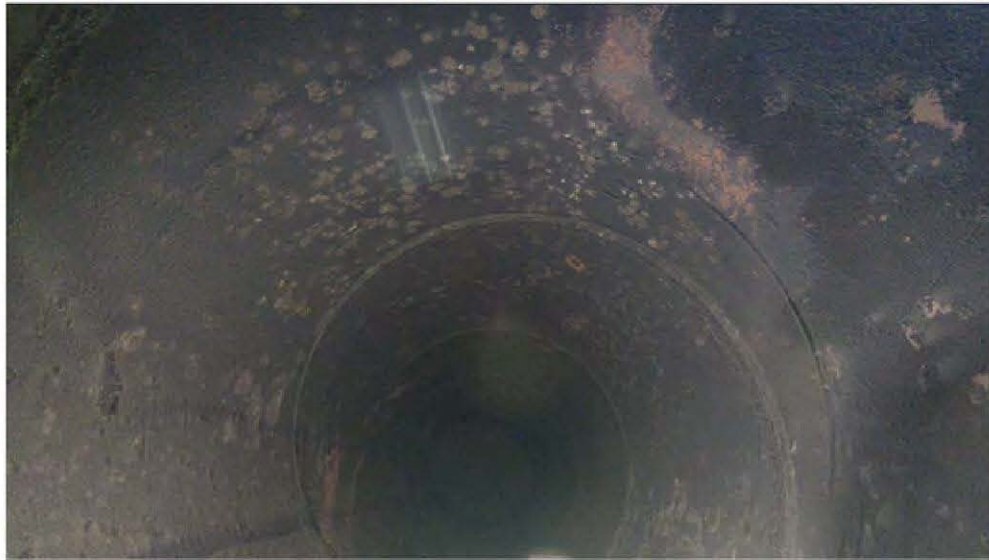
Photo 2: Widespread pitting throughout ventilation line.
