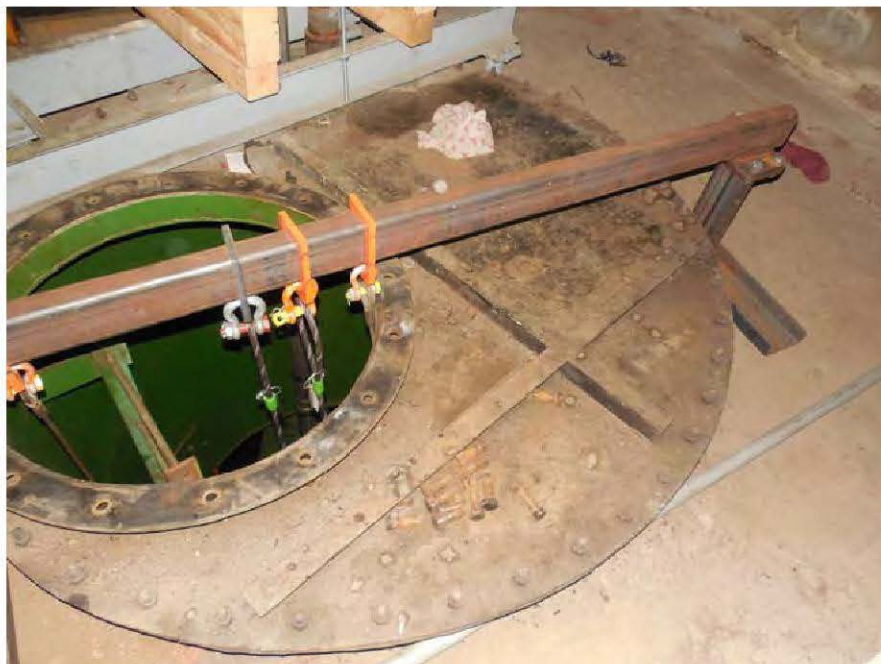
Photo 11: Support structure and cables for spider basket.
