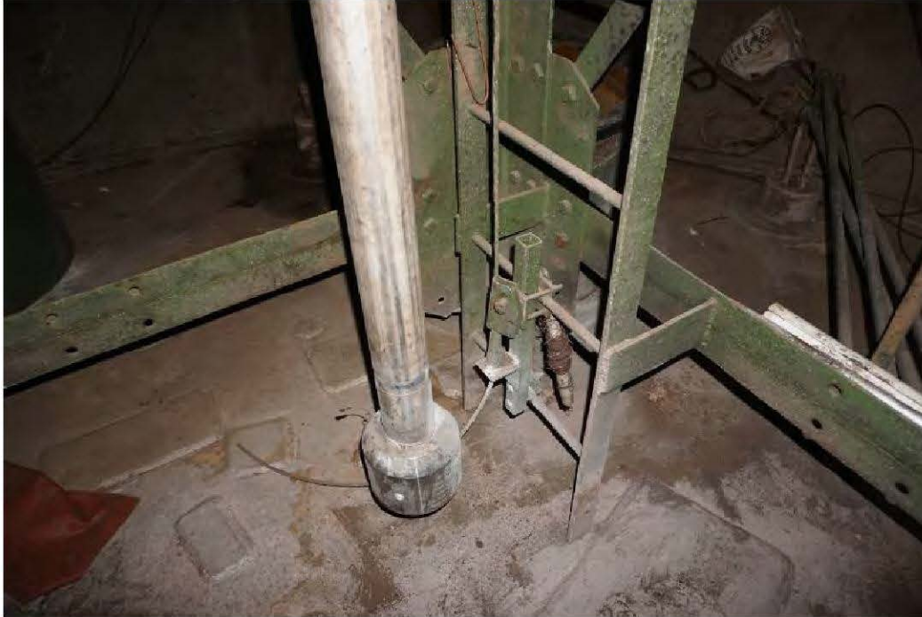
Photo 22: ATG at tank floor.
