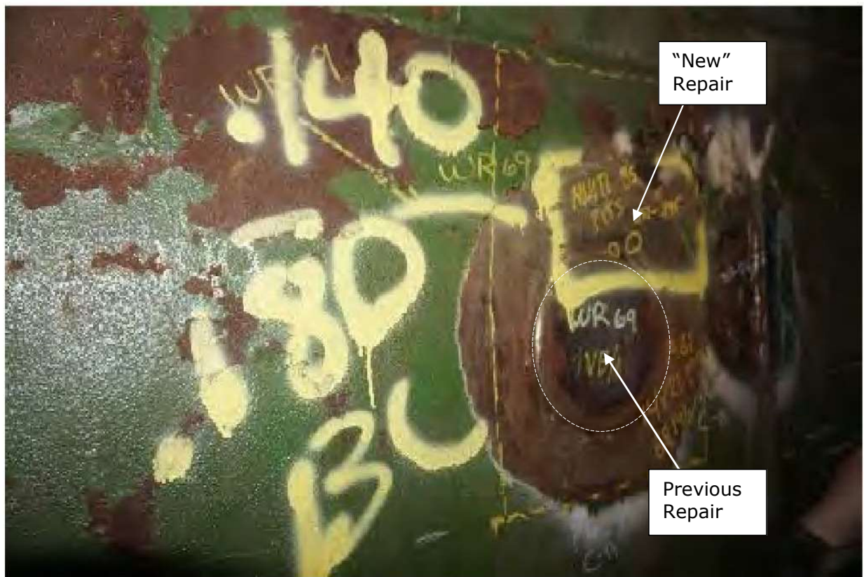
Photo 29: Backside Corrosion around existing patch plates
