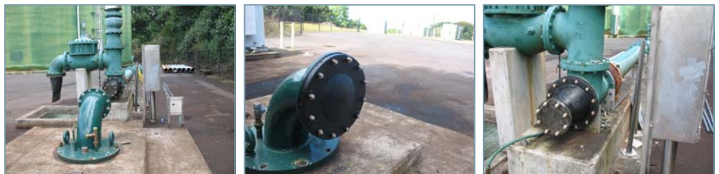
Examples of PROPERLY secured and protected wellheads.
