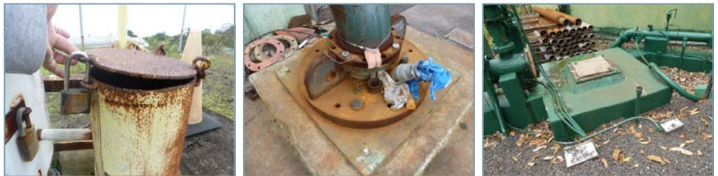
Examples of IMPROPERLY secured and protected wellheads.
