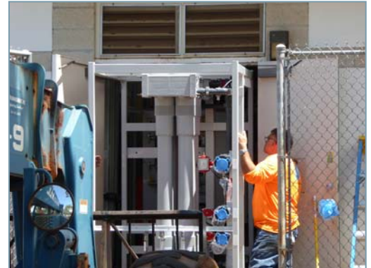
The new Evoqua unit fits through the door at the Mililani Memorial water treatment plant with less than an inch to spare.
