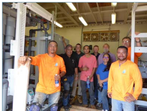
Certified Water Management operators, ITC Water Management contractors, and Evoqua manufacture representative stand beside the newly installed membrane system.
