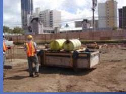
OK Secondary Containment No Overhead Cover
